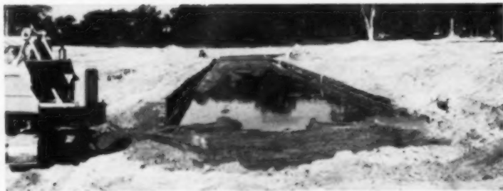
THE BEGINNING —A crane excavates the canal and deposits muck on banks as fill for houses. Total 40,000-yd. excavation cost: $5,600.
