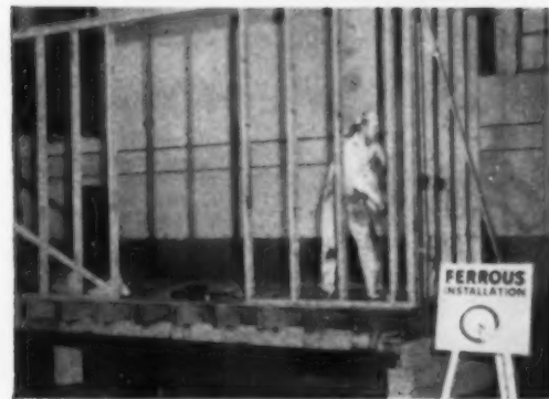
END OF A DAY'S WORK —Copper tube system 100% complete and tested in 7½ hours...less time than installation of only the ferrous drainage, waste and vent lines.
