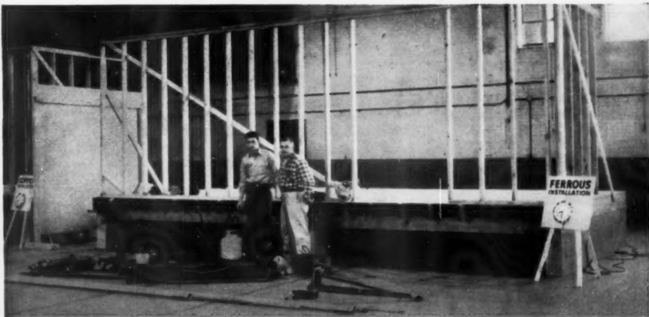
READY TO GO —Teams of plumber and helper, all necessary tools and system components assembled just before start of side-by-side test installations made against stop watch.
