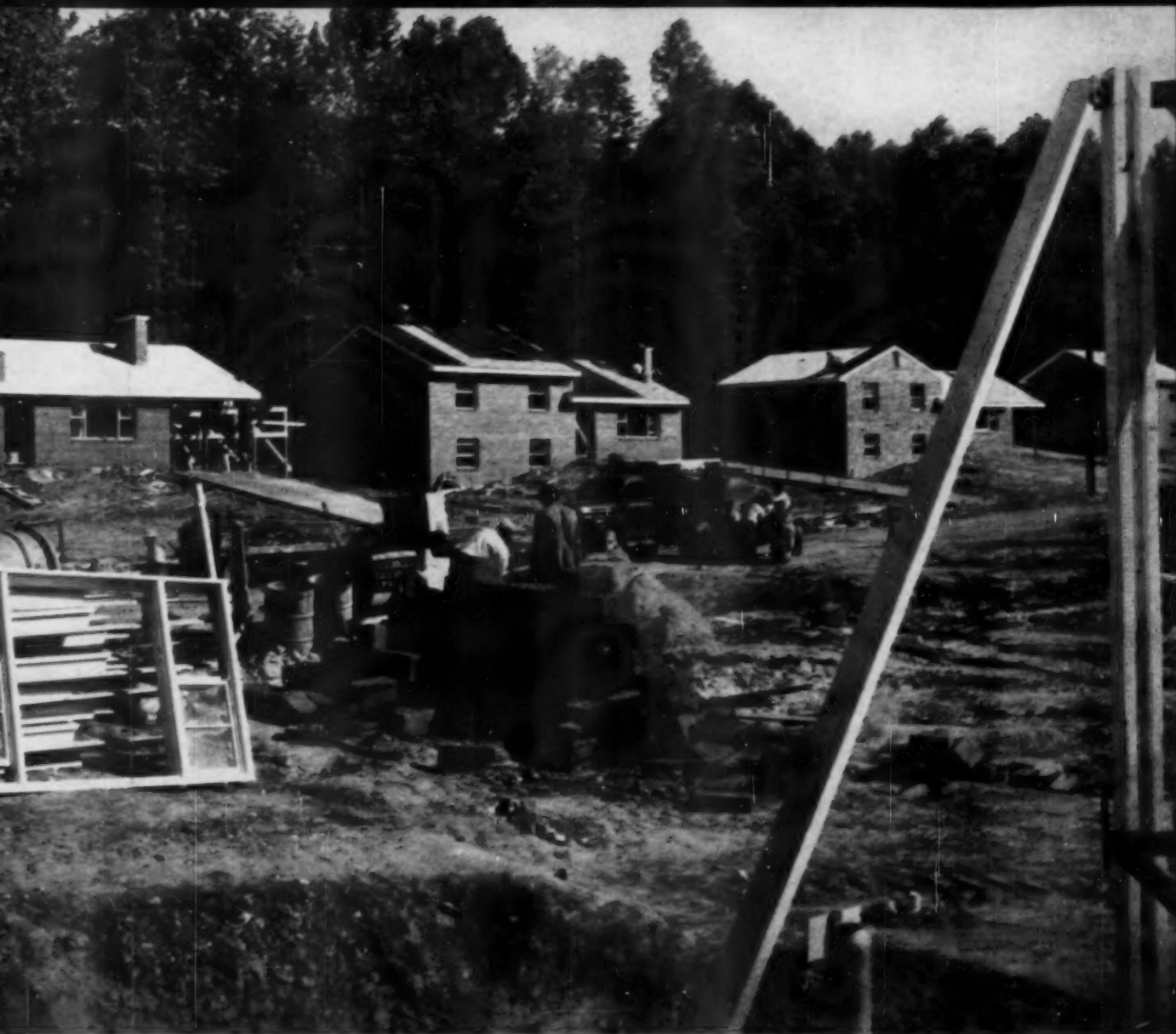
Builders Eddie Carr and Tom Cary can offer masonry houses with basements for less than the cost of prefabs on slabs.
