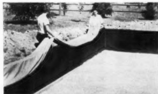
SPREADS LINER NEXT —After bottom of pool is rough graded, sand is added. Then the bottom is fine graded, the walls sealed. Vinyl liner is spread next.
