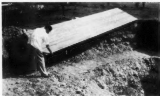
THEN ERECTS WALLS —Specially-treated Wolmanized wood panels make up pool's side walls. They're locked in place after back hoe digs hole to specifications.
