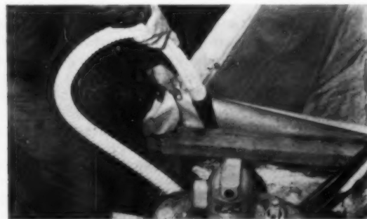
AND PULLS LINER IN PLACE —This machine creates a suction that pulls the liner into place, and makes it possible to do the complete job in a single day.
