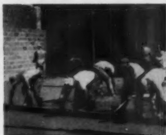
FLOATING —Work crew strikes concrete off, then bullfloats it to a rough finish. Slab is 2½ in. thick.
