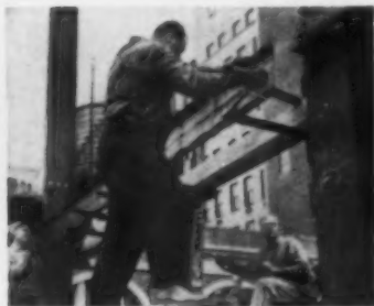
ERECTING —Girders fall into place, hand-guided by workmen. This starts structural phase of 3-story job.
