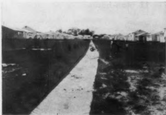
4-FT. CONCRETE SWALE runs between back yards. It's flush with the ground, doesn't interfere with use of the yards.
