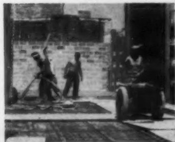
CONCRETING —Workmen buggy concrete onto reinforced deck while one man vibrates concrete.
