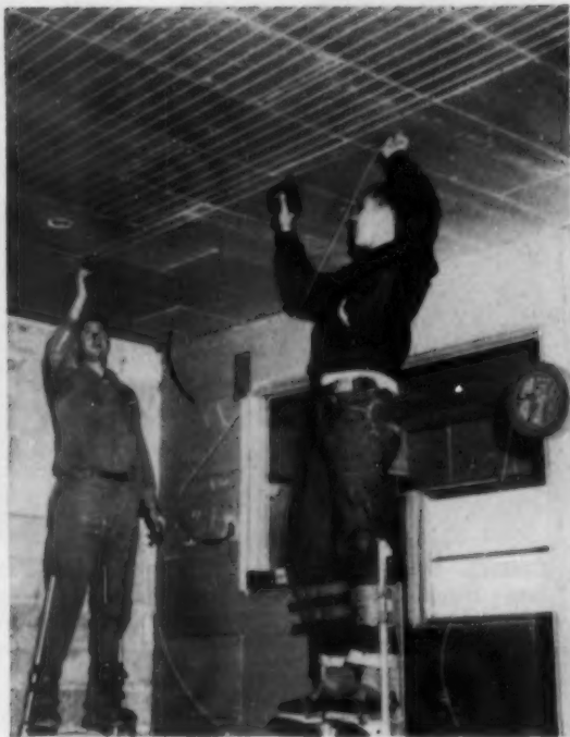
RADIANT CEILINGS —Workmen atop stilts fasten cables to ceiling in parallel patterns. These are covered with plaster or drywall. Method makes ceiling a radiant panel that sends infra-red rays down over the room.
