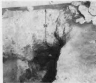
PITFALLS? . . . can be many, says McGee. Plumbing sub had to knock out unexpected 28" of concrete.
