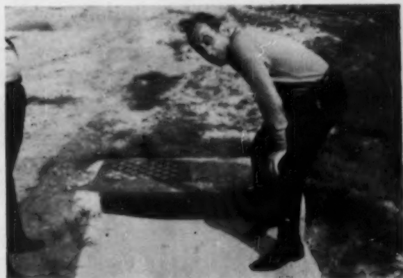
CATCH BASIN at end of the swale collects runoff. If the drain clogs the runoff is distributed, to minimize erosion (sketch, left).
