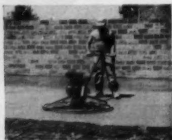
FINISHING —Timesaving mechanical finisher smooths floor. Adjustable blades make different surfaces possible.
