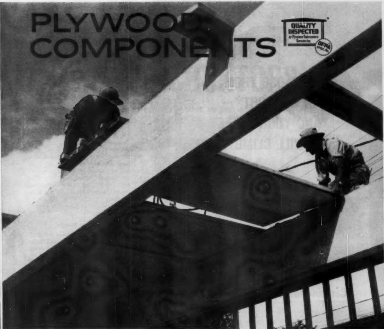
In building at Rochelle, Illinois, Hines Box Beams span 35'. Stressed Skin Panels form roof deck. Architect: Gene C. Jackson.
