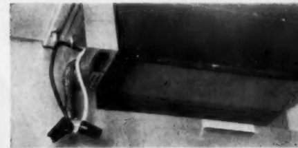
Only two wires connect to house line
