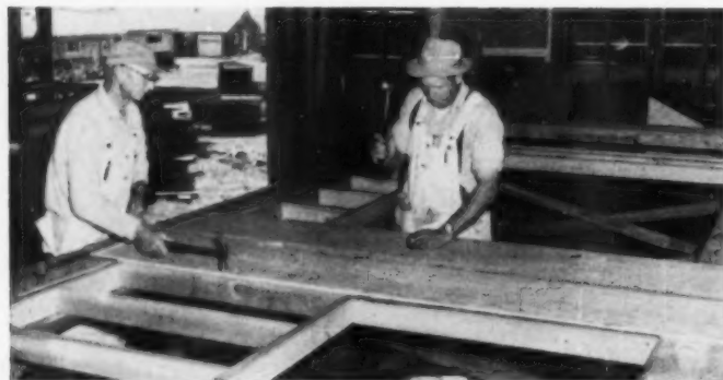
TWO MEN apply insulated sheathing, building paper, and siding. Horizontal siding is site applied; shakes, or board and batten, are shop applied.
