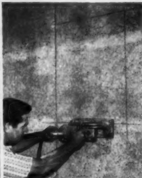
Wall sections are set solid and openings are cut out with Skilsaw quickly and easily.
