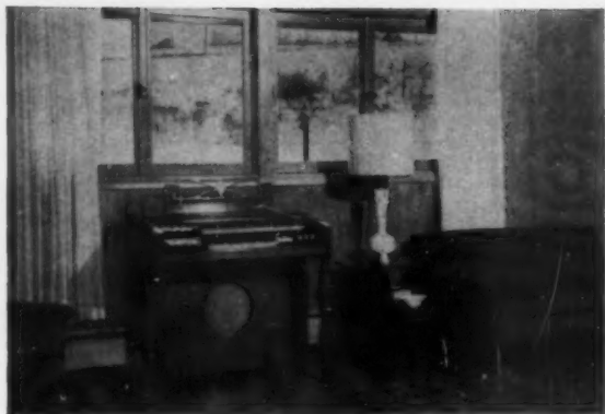
All upstairs rooms, except dining room, are heated with Chromalox electric baseboards.
