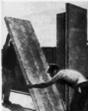
Tilt-up wall construction technique for fast wall assembly with only two men.
