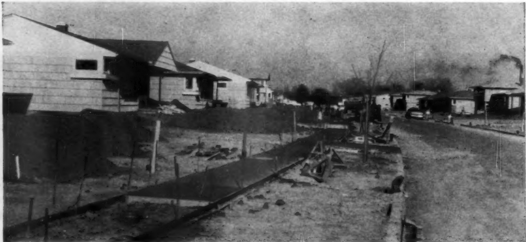
DOWN THE STREET —house-by-house—grading, sidewalks and approaches are completed along with the exterior painting.
