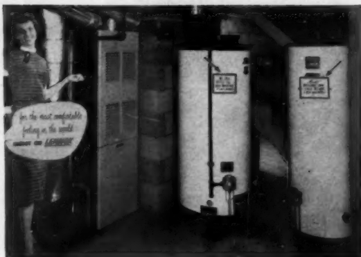
DISPLAY in basement of model house consists of eye-catching stand-up model. Note two water tanks to dramatize economy, longer guarantee of larger tank.
