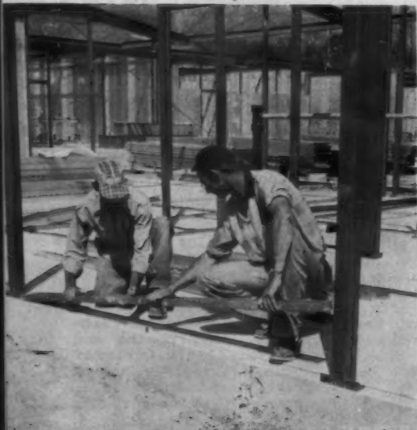
STEEL CHANNEL: this is where exterior panels are set with fastening bolts. These can be removed, making the building portable. Floors in the school are concrete. If and when the building is moved, the concrete can be left at the site and used as a play area.
