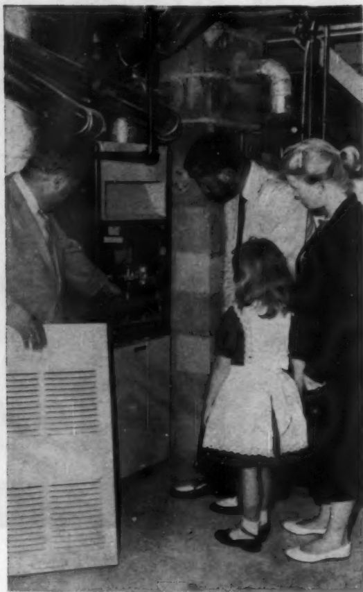
DEMONSTRATION by Loving sales manager Peter Chakeres points up advantages of Lennox warm-air furnace to prospective home owners. Chakeres gets man into the act by having him actually operate the mechanism.
