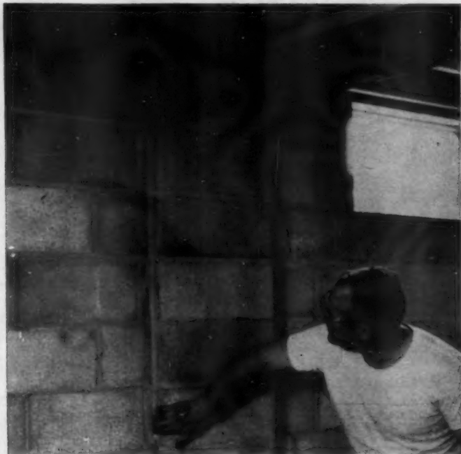
CONCRETE block pilaster was designed by Pearces to eliminate cave-ins during winter building. It works perfectly. After block is set, center well is filled with poured concrete. Al Stange checks it here.
