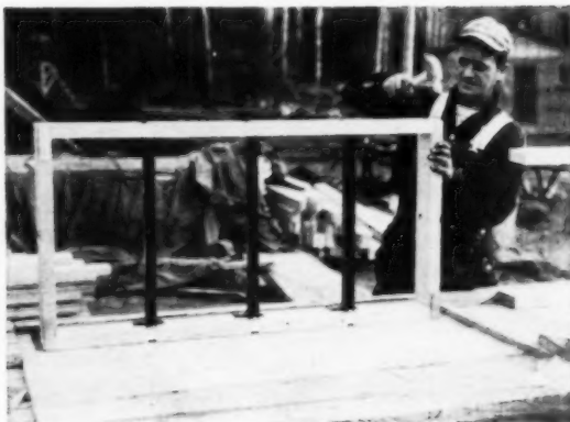
MAINTENANCE. You don't always have to build a new frame to keep the form in service; one nail may do it.
