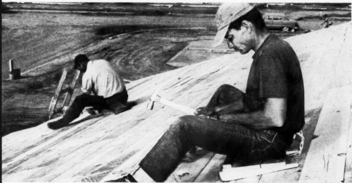
•• My favorite time saver! These little wood 'scooters' are used by crew in nailing roof
