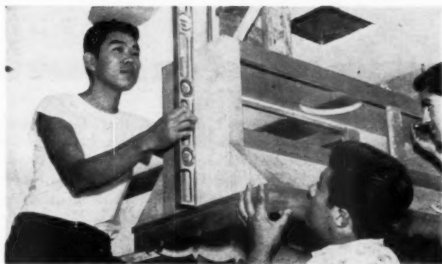
STUDENTS at L. A. Trade-Technical Jr. College complete work on the Campus Home. The house
