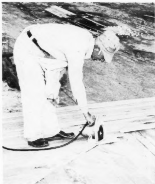
““ Roof boards are laid in place loose by laborers, then trimmed off by carpenter before nailing.”
