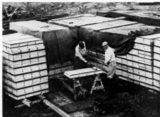
CLEANING and storing. After forms are cleaned and oiled, place in dry place with slight pitch for run off.
