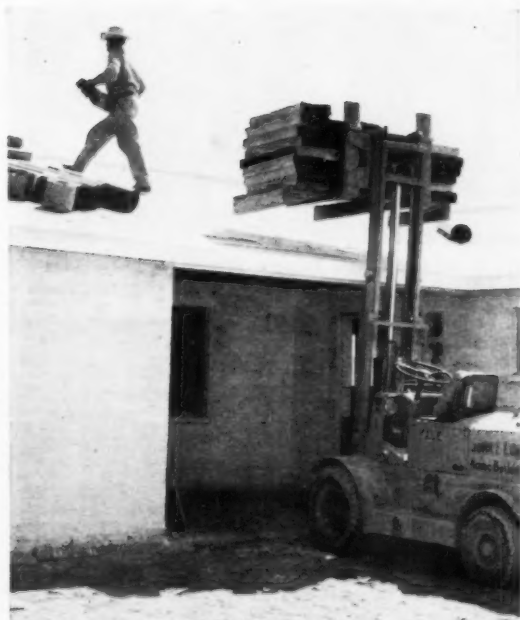
•• Another time and money saver: roof shingles are hoisted with this fork lift, spotted by laborer on roof right where they will be needed."
