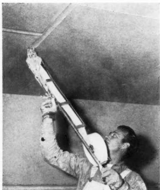
““ Taping machines like this cut time 1,000%. Our two-man crews have it down to a system, take 45 minutes to tape a house instead of one day”.
