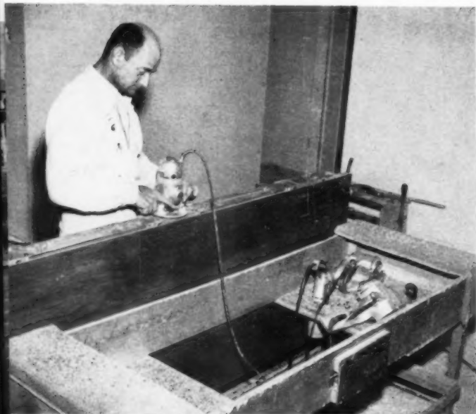
““ This handy jig workbench is a time saver: two-man team installs 70 doors a day. They do a precision job with router, template, joiner.”
