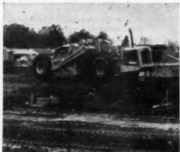
Here Tournapull spreads excess material to grade for housing project near Columbus.
