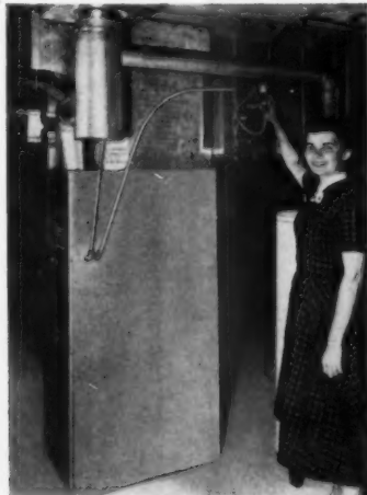
HANGING from basement ceiling, Bryant "Suspendaire" fits plenum in Shelbyville, Ind. home. No. 8004.
