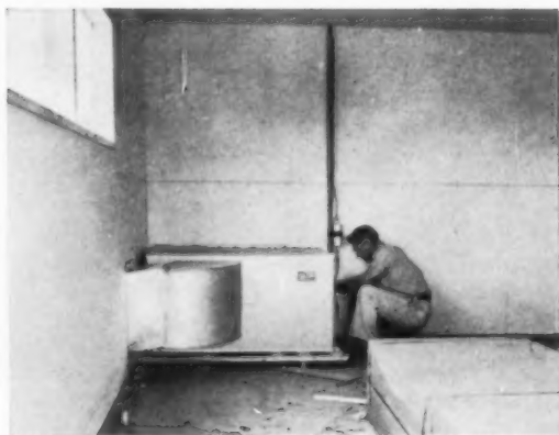
2 CARRIER COMPRESSOR unit is installed in the back of the garage, cooling air comes through holes in the wall. Ductwork is kept to a minimum. Garage is 25 ft. long, leaving plenty of room for cars.
