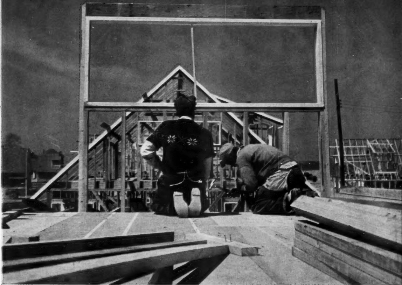
GABLE END SECTION , with window frame installed, goes up. Note that in fully-framed house (background),
