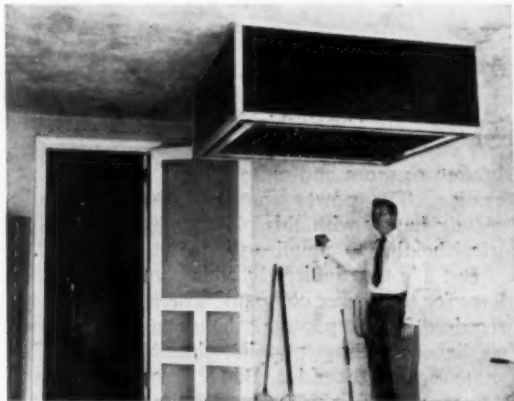
WARM HOUSE AIR is exhausted through attic by double-duty Lau fan job in Louisville. Garage door is closed.
