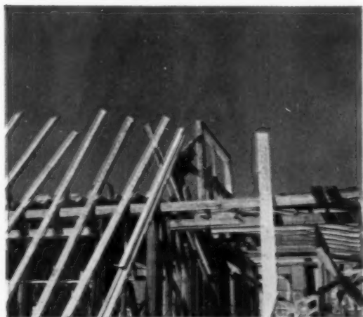
RAFTERS , precut and notched, are laid against side of house ready to be sent up. To this point, all houses are the same; from here on, roof lines on the house and garage are varied slightly to avoid "cookie cutter" look.
