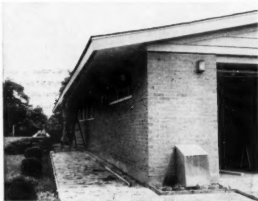
SOFFIT LOUVRES help gables promote thorough air change, prevent stratification in this garage fan installation.
