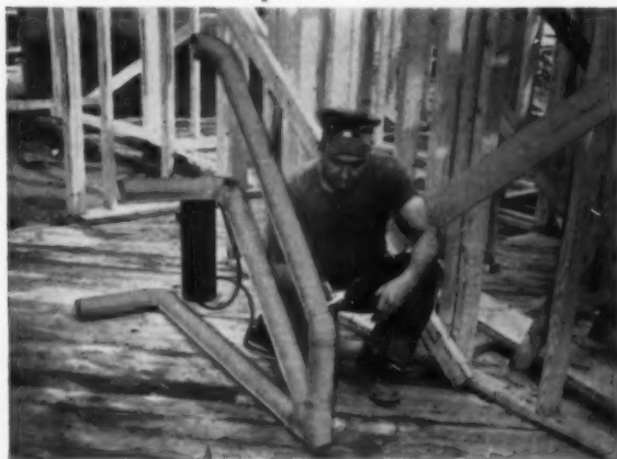
Prefabrication —"This double-Y and other sections can be pre-assembled out in the open or at the shop where men can work easier and faster—no lost time waiting for construction."
