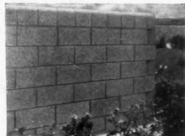
Note the uniform texture and straight, sharp edges of this beautiful concrete block wall.
