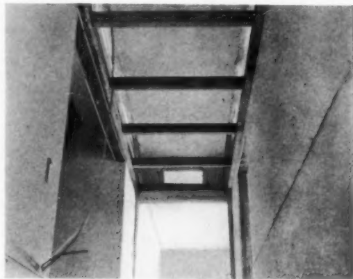
4 HALLWAY CEILING is dropped and covered to make cooling duct for the bedroom wing. This method is used where duct runs at right angles to joists. Where they are parallel, duct is set up between joists.
