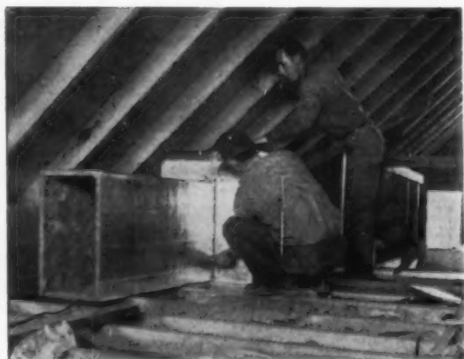
1 GLASS FIBER DUCT covered with aluminum foil is shipped flat, assembled quickly with tape, adhesive. Duct is installed far to one side where it won't interfere with later expansion of the attic.
