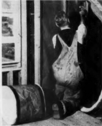
Hansen Tacker tacking insulation—one of many uses in doing a faster, better job, and cutting costs.
