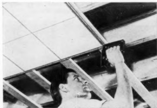
Celotex Tile Board ceiling is stapled to furring strips. Check reply card No. 7035, p. 148.
