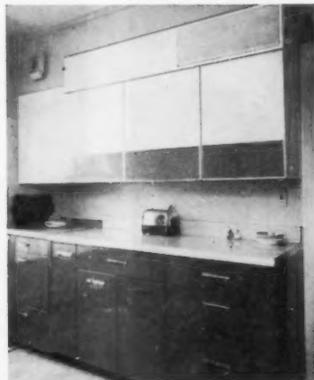
◀ AFTER installation of wall-hung refrigerator, which hangs on a 5-foot mounting bracket bolted to wall studs. Unit is 64" long, 39½" high and 17½" deep. Check No. 7071 on card, p. 148.
