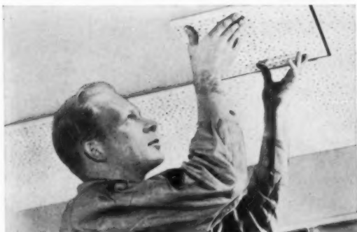
Armstrong Acoustical Ceiling Tile is being attached with adhesive. Check reply card No. 7033, p. 148.
