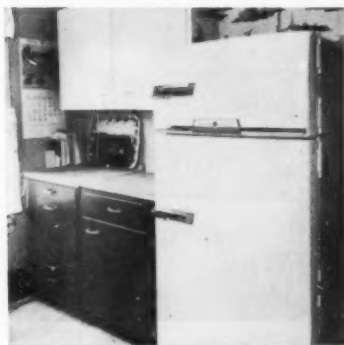
BEFORE: Installation of new General Electric wall refrigerator, one wall of this kitchen looked like this.
