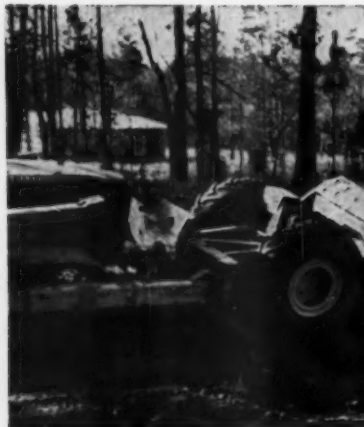
7½-yard Tournapull shaped backslopes while grading roads around Mauvilla subdivision, also leveled and sloped land for drainage.
