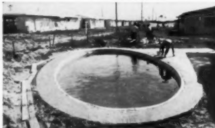
1 NEAR COMPLETION , this Florida job by De-lorich of Miami shows skirt of concrete.
