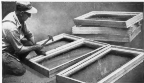
Shop assembly of Flexivent Units into larger window groups is method used on Rolling Hills project. Assembled units are trucked to building site as needed. "No unit so easy to stock as Flexivent," says Mr. Kramer.
