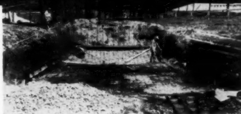
Excavation for pool showing steel reinforcement for floor and inside pool walls.
