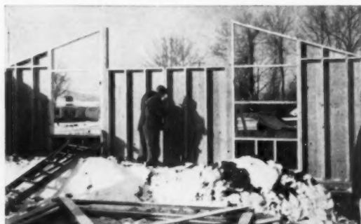
4. INSIDE VIEW OF GABLE END clearly shows panel system. Four by four posts in wall hold roof girders; one at left will be sawed off. This is start of the second day, when the sun decided to come out.
