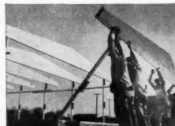
Contractors R. A. Koplow and I. W. Konigsberg erected these twelve Rilco post and beam frames in one hour. Pitched beams spaced 6' o.c. have a clear span of 21' 6" with a 3' 6" overhang.
