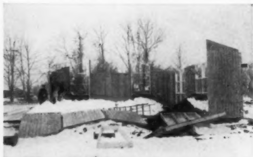
3. WITHIN TWO HOURS of raising the first panel, house has reached this point. Work on the first day included unloading the truck, was done in a blinding snow and hail storm, still went fast.
