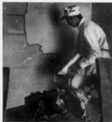
A. W. Peterson, plastering contractor for M. J. Peterson, Inc., says that Lite-Mix is stronger and has a uniform suction. Here Lite-Mix Plaster is being applied over Certain-teed Beaver Gypsum Lath.
