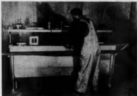
OPERATOR is shown here planing door on the hinge side. The plane has attachments on it to control the bevel exactly and also to size the door perfectly. After planing is finished, next step is to use combination door and jamb stop.
