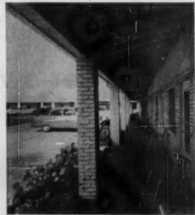
COVERED PORCH provides sheltered promenade in front of all units. Unfinished ceiling, rough brick, give a ranch house flavor.
