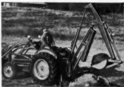
LOWERS EXCAVATING COSTS —Ford Tractor and backhoe is ideal for digging footings, bell holes, laterals and septic tank holes. Easy hydraulic operation. Compact for maneuverability.
