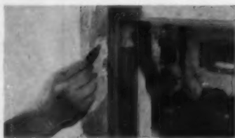
FELT SASH PLUGS are installed at the point where meeting rails meet.
