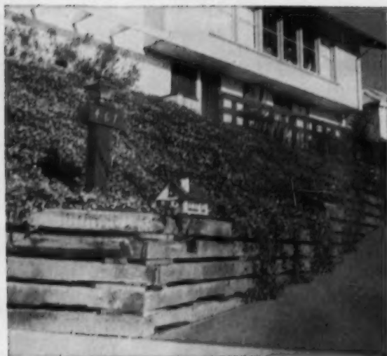
Railroad ties (illustrated here), redwood logs or pine battens used as cribbing will retain earth fill where slope conditions call for medium to high devices
