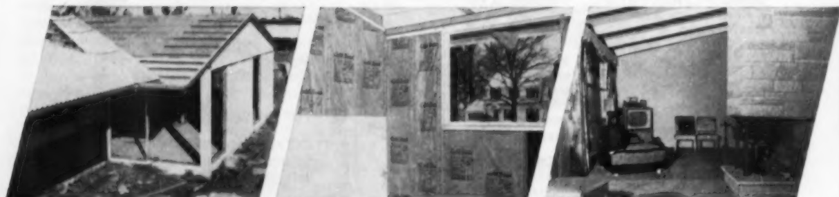
Two men nail on permanent roof of Gold Bond Economy "250" Corrugated Asbestone, while third man nails Gold Bond Gypsum Wallboard to purlins from interior.
