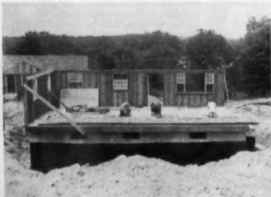
2 Wall sections are built flat on the rough floor, using it as a foundation. Then exterior wall shingles are applied and windows installed. The full wall sections are then tilted up into place.
