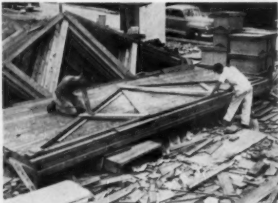
5 Simple 2 by 4 trusses with a 24-foot span are built on a platform at the site. The truss eliminates need for load-bearing partitions.
