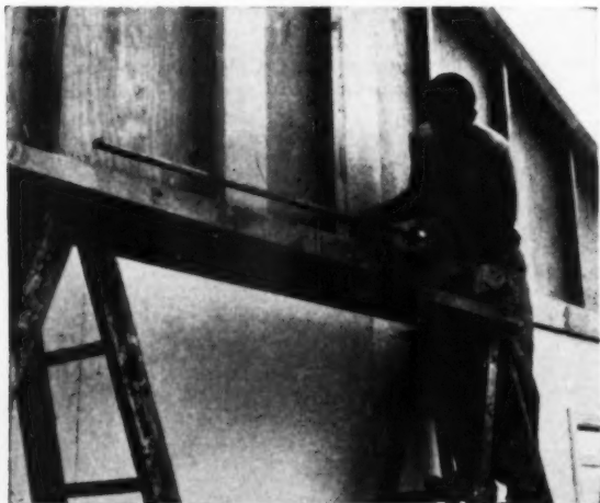
A clamp is used to pull two gable end units firmly together before nailing
