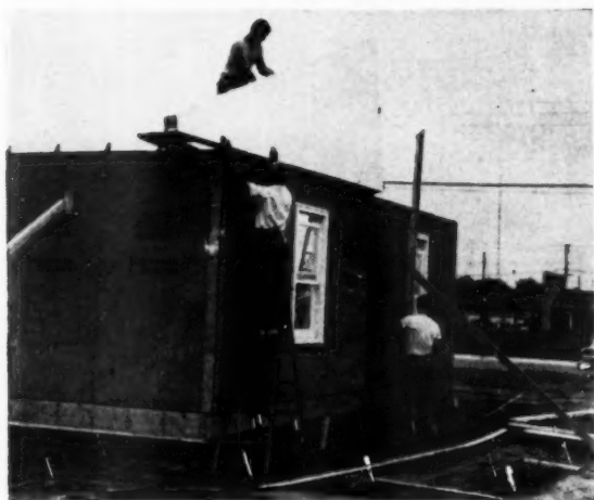
Gable ends are fabricated in two sections to minimize weight, speed handling
