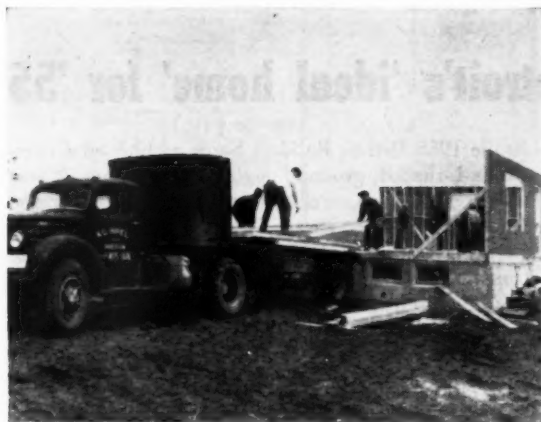
Picture above shows N. O. Hipel shipment of prefabricated panels to site of builder customer. Walls, trusses and roof decking can be erected in one day
