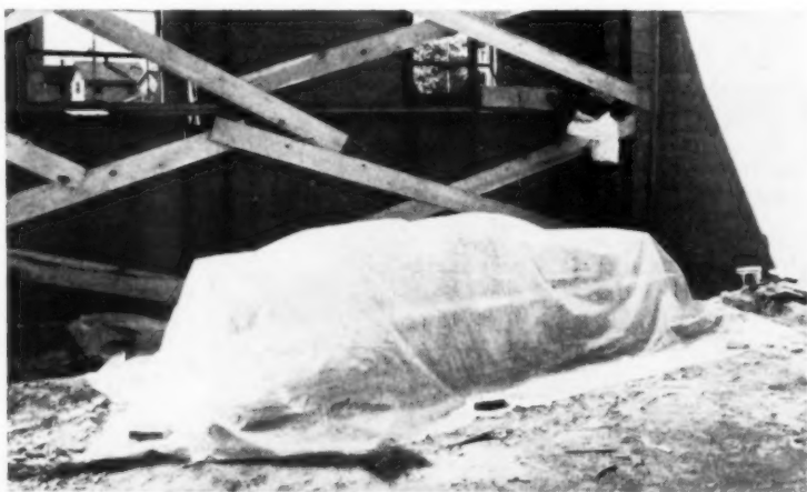
Film can be used as a tarpaulin over lumber. This can apply to machinery, cement, and other building materials
