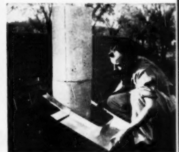
Aluminum flashing is installed on the roof. Van-Packer's "Brick-Panel" Housing over its aluminum flashing gives chimney a weathertight seal.
