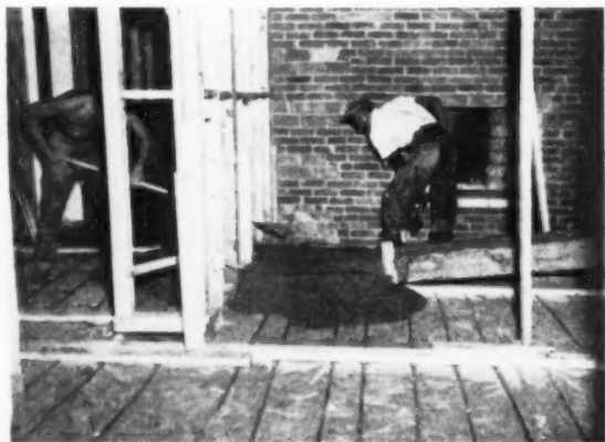
Radiant heat piping is shown laid over a moisture barrier film preparatory to the pouring of concrete
