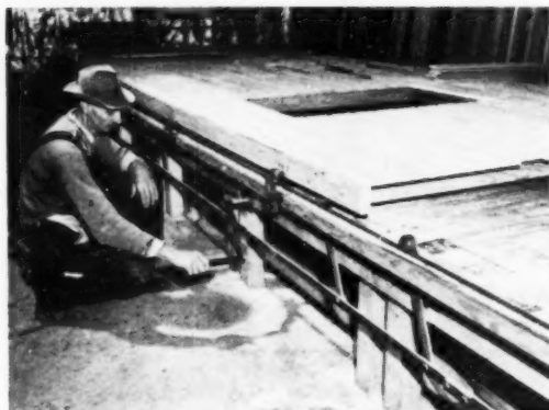
Step No. 5. It takes 5 to 8 seconds to raise the frame assembly to roll it down the line for further processing or removing from Erector
