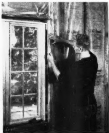
Applying scotch tape to jamb of window opening which holds the film in place until the room surface material is installed
