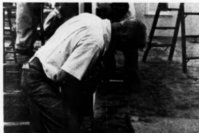
A three-inch screw is driven through bottom plate of panel into raised floor plate. Workman uses 1/2-inch drill and power screw driver
