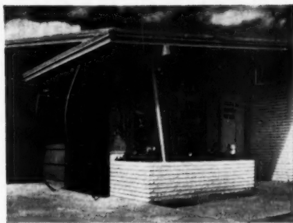
Here a vertical roller awning is used in conjunction with a west overhang that cannot provide complete protection from the low late afternoon sun. Not shown are matching gray and green striped standard awnings; shielding east windows, which are an equally critical source of heat.
