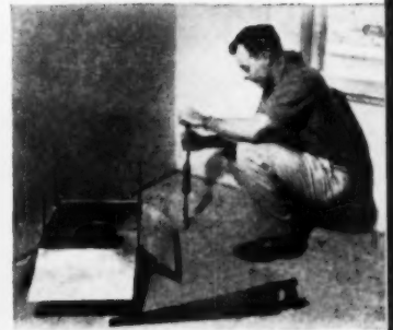
Openings quickly prepared in the floor, for the chimney support, and in the ceiling and roof to permit passage of flue (floor suspended method).
