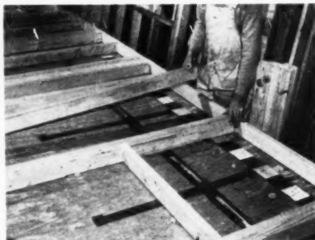
Step No. 2. Setting studs in stud locators. Change over from one side of house to another is simple
