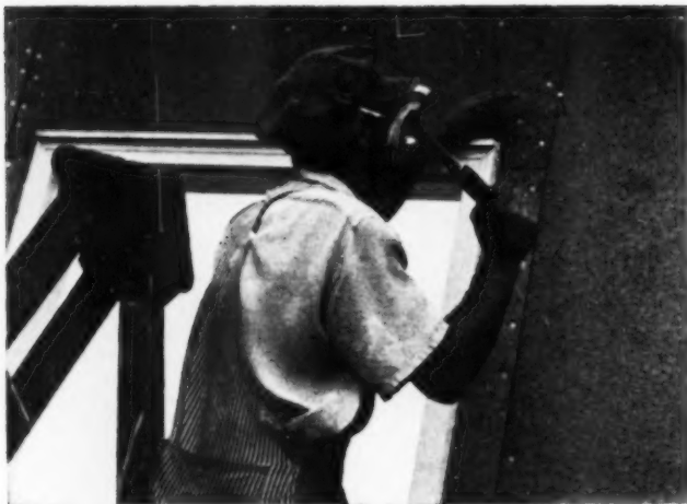
Carpenter drives a 16d nail through exterior insulation sheathing into built-up post
