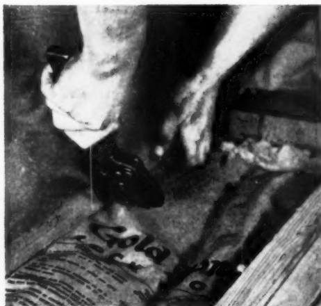
Vapor barrier stapled in place at ceiling line. Staples with \frac{1}{4} to \frac{3}{8} -inch legs should be used at 6-inch centers. Film should be stretched fairly tight across the studding
