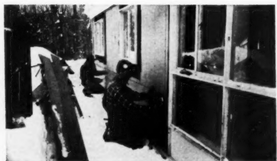
Siding should be pre-primed on both sides before applied. Siding in photograph has been dipped in stain before application
