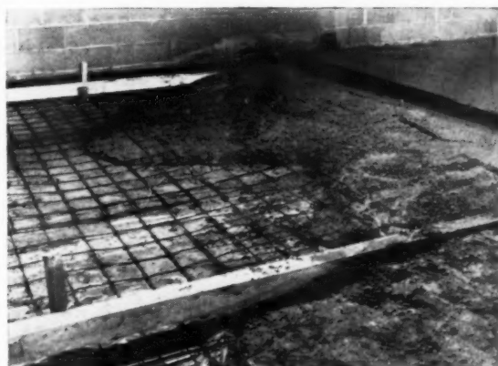
Moisture barrier in position under reinforcing mesh. Concrete is poured with mix spread in the direction of the laps
