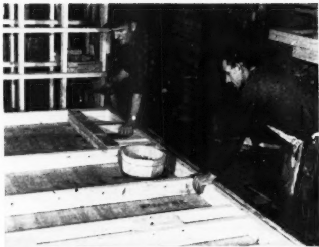
Setting up a modular panel system based on an American Builder series of articles, two Canadian building firms operate central cutting and fabricating shops; ship to job. Picture above shows shop of Roy James Construction Co.
