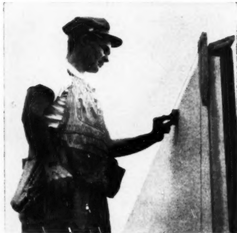
A line is used to straighten the wall as the trusses are installed. Corners were plumbed and braced previously
