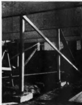
Frames rest in steel pipe sleeves set in piers. Sleeves are grouted when the slab is poured. Posts are treated
