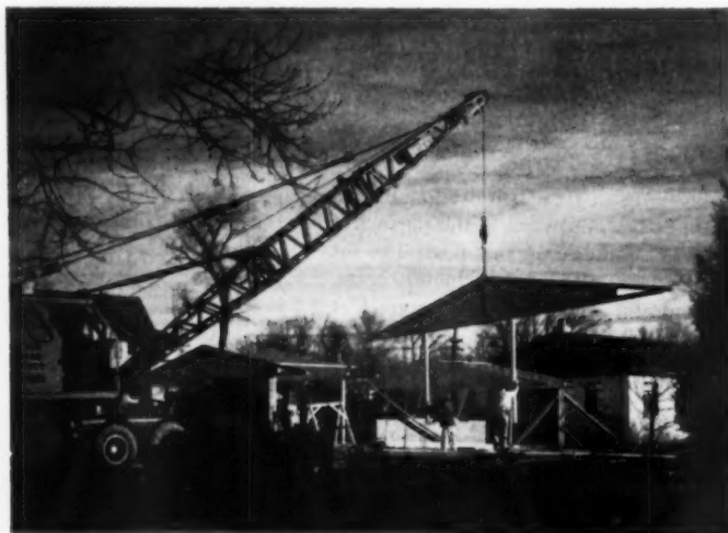
Posts on this frame show the cantilever possibilities. Actually, the longer cantilevered length is 21 feet. The deflection after the roofing was applied is less than \frac{1}{8} -inch
