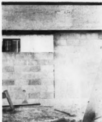
Exterior masonry walls were laid up in panels. An expansion strip was inserted between units, and \frac{1}{4} -inch rod was imbedded in the mortar every third course, reducing tendency to crack
