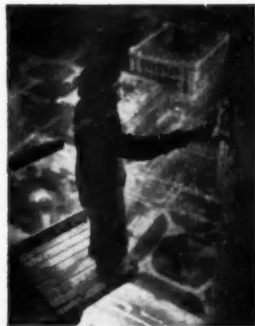
Photograph on left shows how Bob Reynolds, of H. Reynolds Company, of Cleveland, Ohio, stands on extreme edge of hanging scaffold, 614 feet above sidewalk.
