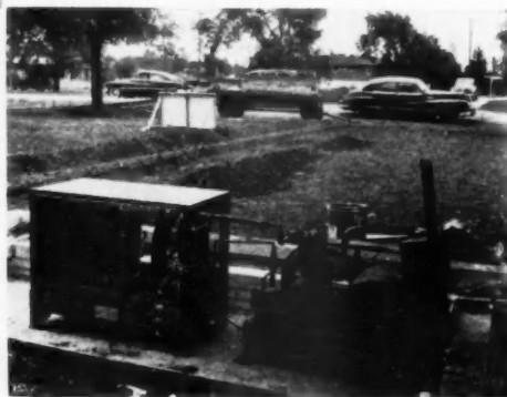
Condenser and compressor are installed in outside housing, leaving much inside space for other uses. Surrounding planting area for shrubbery is intended for attractive landscape feature minimizing location of the box
