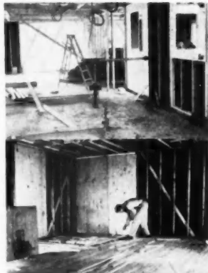
Absence of bearing partitions simplifies rough plumbing and electrical work, saves estimated 30 per cent labor cost in flooring and wallboard application
