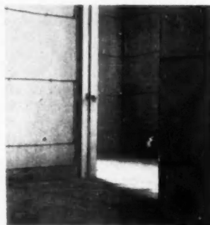
Partitions before plastering. The \frac{3}{8} -inch thick plaster-board rests on a wood bottom rail, which acts as a skirting for both sides of partition. Reinforcing wires are held by hook nails driven into the surrounding frame
