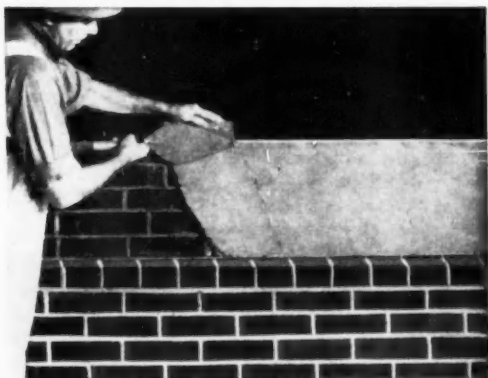
The face brick should be backplastered.
