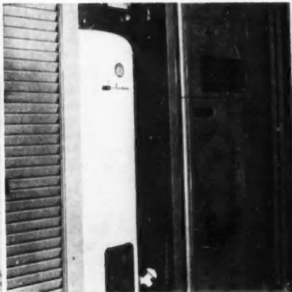
Water heater, gas furnace, with cooling unit above, fit in small closet space
