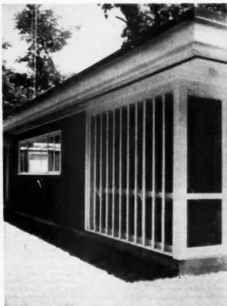
Porch louvers break view from adjacent busy street. Porch floor is a scored concrete slab. Continuous vent is under soffit
