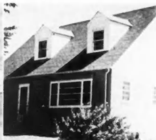
day afternoon between 2 and 6 p.m. The next morning at 7 a.m. he found the paint blistered as shown above. The blisters are hollow and contain no water. The siding and woodwork were thoroughly dry when the blisters formed and when the photograph was taken a few days later. Testing on houses afflicted with temperature blistering has shown that the moisture content of the boards was from only 8 to 12 per cent.
