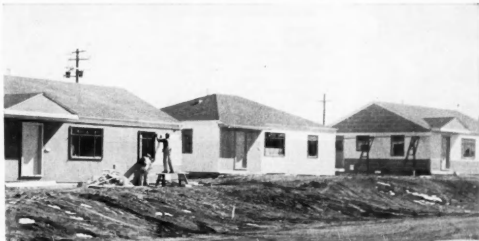
Applying two-tone asbestos siding. First three courses are in one color, remainder in second. Roof matches or contrasts with siding
