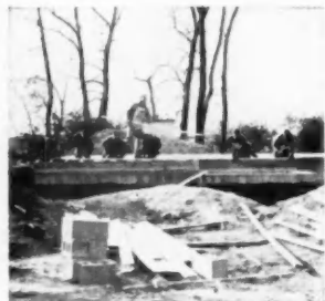
WORK UNDER WAY on students' third house, with plenty of hands available
