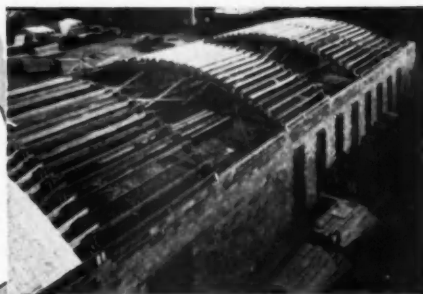
C. T. Hubbel Lbr. Co. Warehouse, Albany, N. Y. Contractor: Koch Bros., Albany, N. Y.
