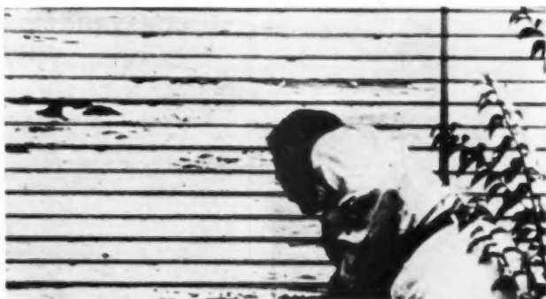
TOO MUCH MOISTURE INSIDE THE HOUSE was responsible for this failure of peeling. The black line divides the kitchen on the left from the dining room on the right. Excess moisture vapor in the kitchen can be removed by installing a suction-type fan in the kitchen window or wall.
