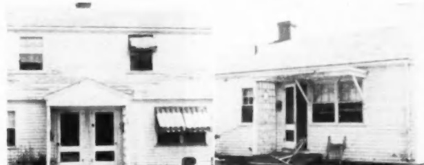
WHEN POOR PAINT BEGINS TO FAIL , the failures tend to be worst on areas that receive most water during storms. On the house at left, the worst scaling is on the siding which is next to an entrance roof on which snow evidently piled up and melted during the winter. On the house at right, the lower courses of the siding show most paint scaling, except where the roof over the entrance furnishes protection. (However, the fascia board of the porch roof has badly scaling paint in accordance with its lack of protection.) Paint on this house did badly on galvanized iron down-pouts because they had not received a good metal primer before the house paint was applied.
