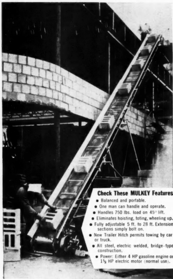
Forty-foot Mulkey carrying 16 blocks per minute to second floor level 23 ft. up.
