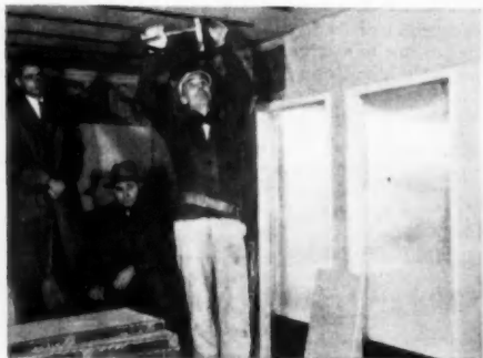
100% GOLD BOND GYPSUM LATH. Bill Baker (left) of Cox & Baker and Robert Dickson (center) Robert Dickson Lathing Co., watch as Gold Bond Gypsum Lath and Stripite are applied in a Cox & Baker Colonial Farms home.
