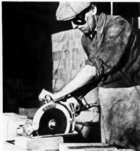
STRAIGHT edge cuts in brick are achieved with the aid of an electric saw and abrasive disc. Quality work and reduction of waste dictate this method in preference to breaking brick
