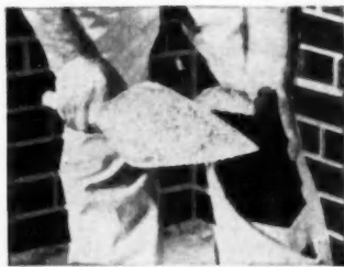
Method 1. Plenty of mortar should be thrown on the end of the brick to be placed.
