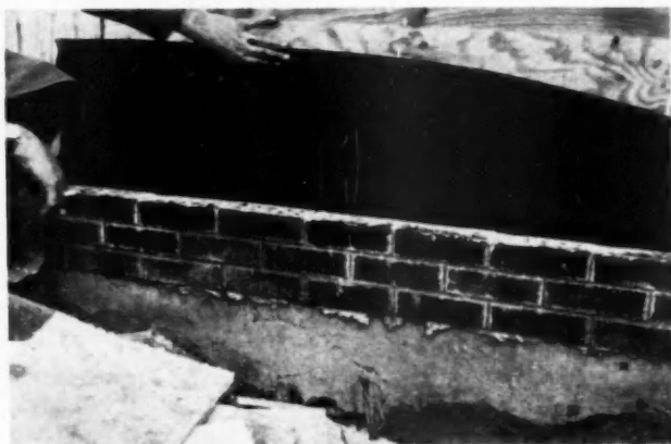
FOUNDATION WALL is poured to grade and one course of 8 inch concrete block laid on the wall. The three courses of brick are visible after back filling
