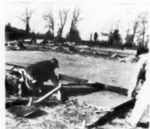
REAR STORAGE ROOM floor finishing is done at same time floor is finished
