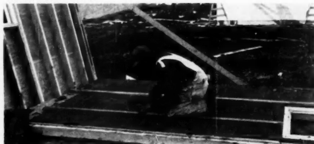
SIDEWALL is constructed in the horizontal position. Framing, sheathing, window and door frames, and siding materials are applied and sidewall tipped into position
