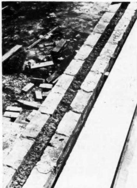
IN THE MASONRY-TYPE WALL CAVITY CONSTRUCTION the type of insulation used must offer good thermal resistance and low density to support its own weight without settling and must resist absorption of moisture
