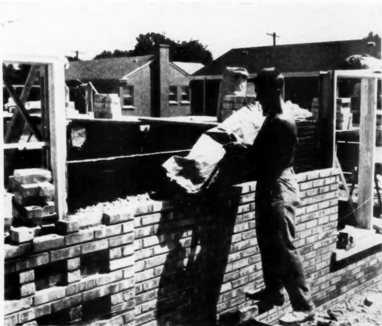
FIBERGLAS CAVITY WALL INSULATION is poured from paper bags containing enough insulation to fill from 37 to 45 square feet of wall with a cavity of 2 to 2½ inches wide. Insulation is poured into cavity when wall reaches window-sill height
