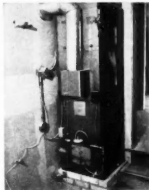
FURNACE in the utility room is raised by the brick work. A sheet metal plenum directs warm air to the crawl space
