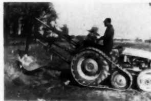
MACHINERY ATTACHMENTS for a tractor reduce the builder's land preparation costs. Here the machine is digging sewer and water lines
