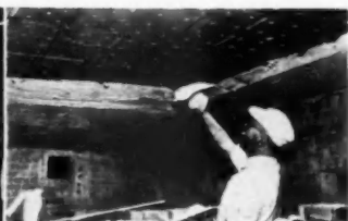
of Standards. Lath is clipped to channels which are tie-wired to open joists; required thickness of plaster is then applied to lath
