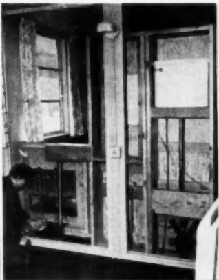
BATH CORE shows the copper plumbing and the installation of water closet
