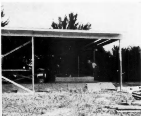
CEILING JOISTS bear on the plywood box girder and perimeter beams. The girder forms the ridge of roof. Finished plywood ceiling is nailed to the joists
