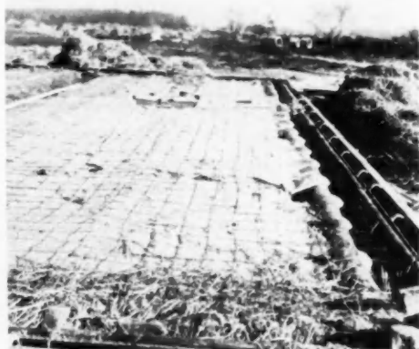
GRADE BEAM FOUNDATION with forms in place ready for concrete. Insulation, plumbing and heating ducts are in
