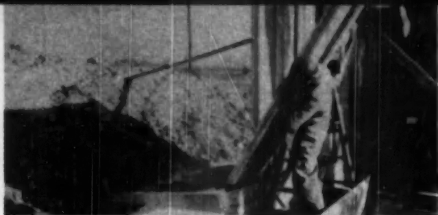
ONE man can handle a Modern-Crete panel. Bottom is held by steel channel
