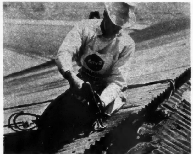
WELDING gun, guided by template, is used to replace corrugated iron roof on old building
