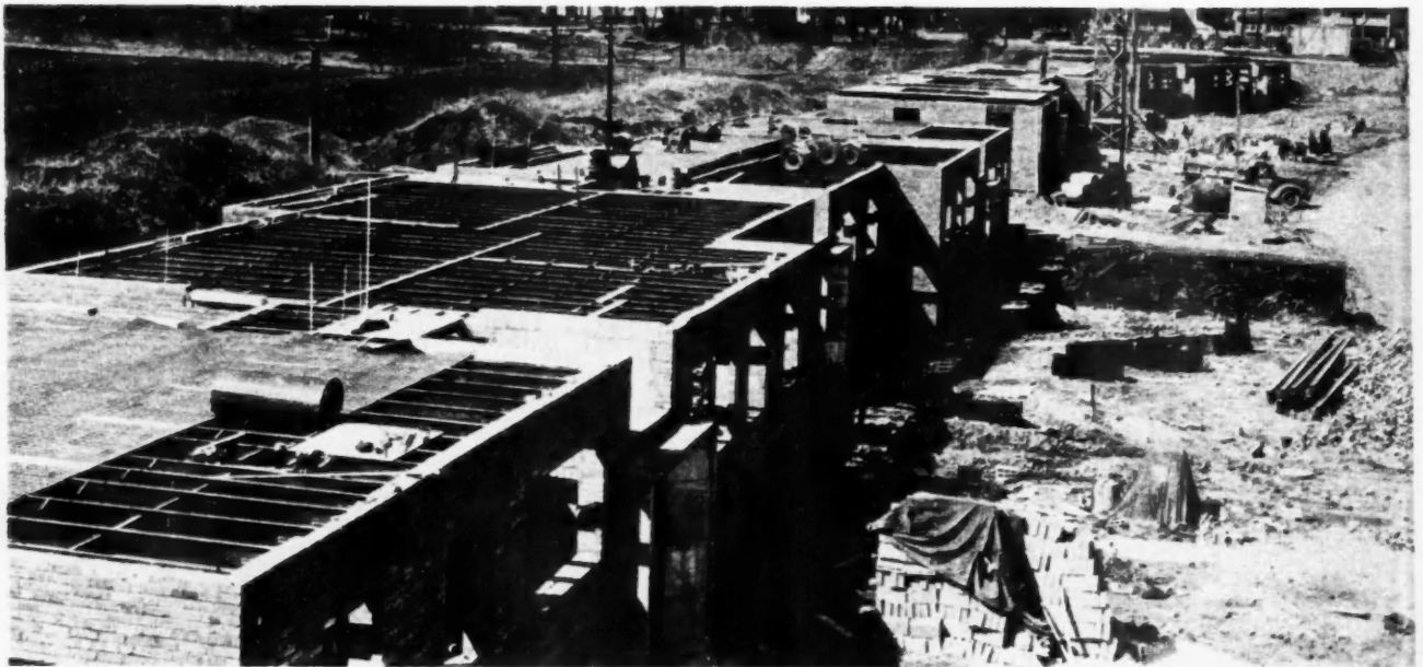
FLOOR lath is placed over 8-inch junior beams before a 2½-inch concrete slab is poured. Beams are spaced 2 feet on center
