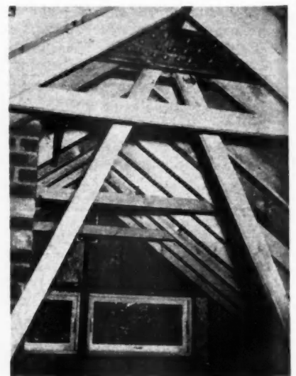
PARTIAL view of roof truss arrangement in the new low-cost Sun Ranch home
