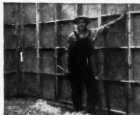
"Seven men set-up the forms for a 26' x 27' basement in one hour and fifteen minutes."—Harry G. Dehring, Carpenter Foreman, Taylor Brothers, South Bend, Indiana.
