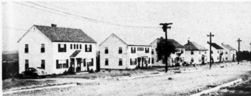
STREETS, curb and sewers were put in the St. Nicholas project by the city as its contribution to veterans' housing project
