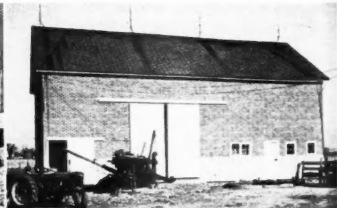
surface for the insulated siding. Insulated siding was nailed to lath furring strips on dairy barn. Completed barn, above
