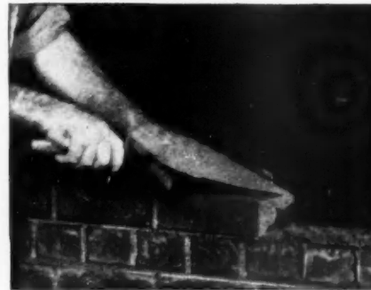
Then plenty of mortar should be thrown on the end of the brick already in place.
