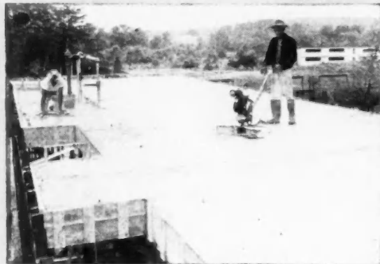
3 Two-inch concrete floor has been poured and finishing operations are under way.
