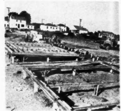
TWO FLOOR panel "jigs", one empty, the other with floor joists and bridging
