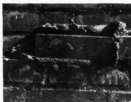
So that the mortar oozes out at the top of the joint.
