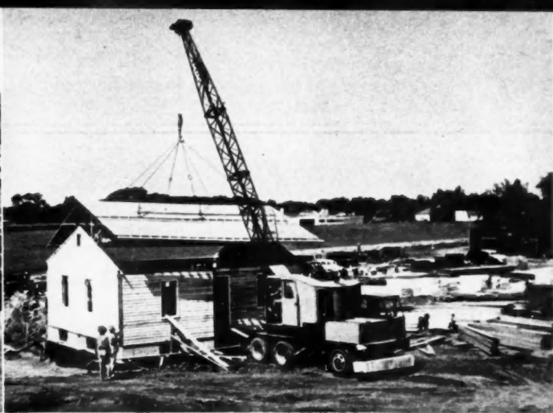
ROOF section being lowered in position on the house. All wall and roof sections fit properly and are quickly assembled
