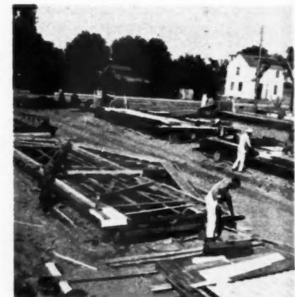
SIDEWALL and gable end of one-story house in process of construction on "jig"
