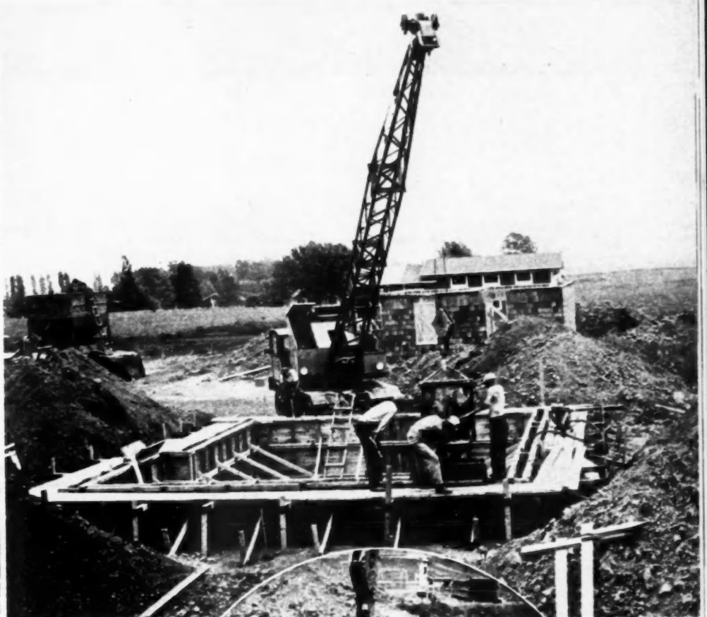
CRANE (work horse of project), swings a large bucket of concrete over foundation forms. Work is accelerated by this method of operation
