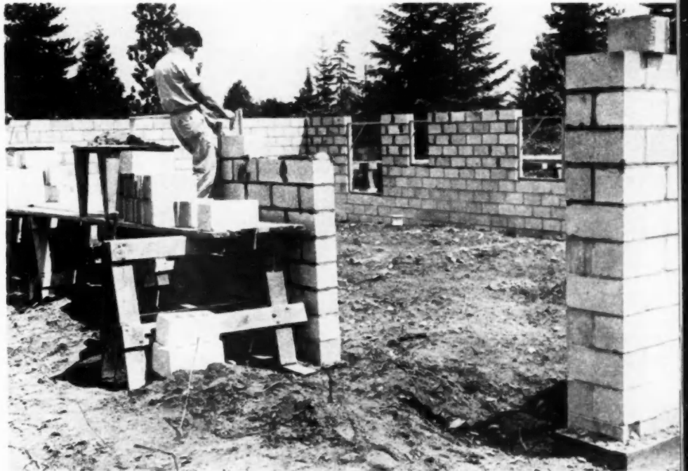
FOUR block layers, three hod carriers lay up one house a day. Block are Graystone "Darex" waterproofed. Outside walls painted; inside furred, rocklathed and plastered.
