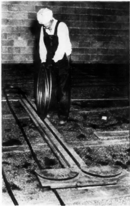
Heat coils of \frac{3}{4} " copper pipe are laid over a 6" pad of washed gravel before concrete is poured. Note wood templet pipe bender. One pipe-man and helper do a house a day.
