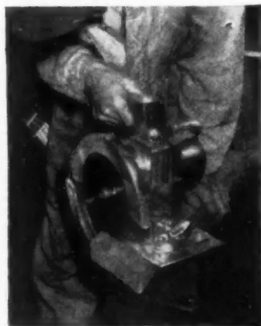
Making a mitre cut following a line can be done quickly and accurately.
