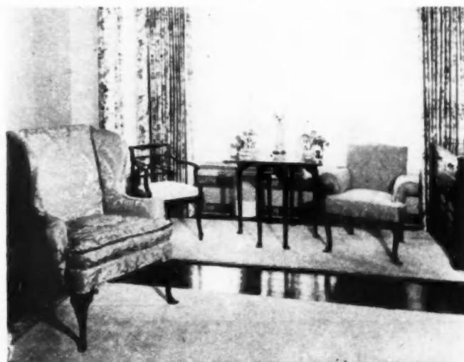
CONVECTOR installation here conforms to curvature of window installation and throws heat upward to counteract cold from glass.
