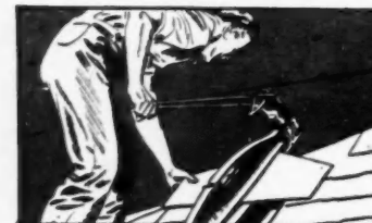
6. Cutter Speeds Application —When shingles must be cut to fit around valleys, dormers, along the rake, etc., a shingle cutter does the job easily, quickly—right on the roof.
