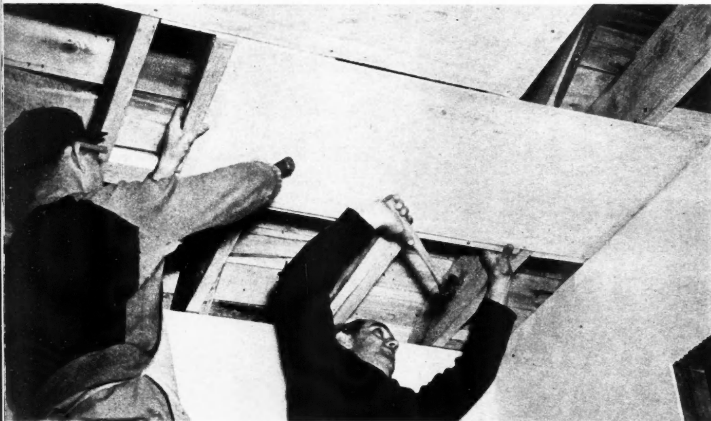
WORKMEN (below) installing panels which may be painted, papered or plastered. Narrow, non-heating border is provided for nailing.
