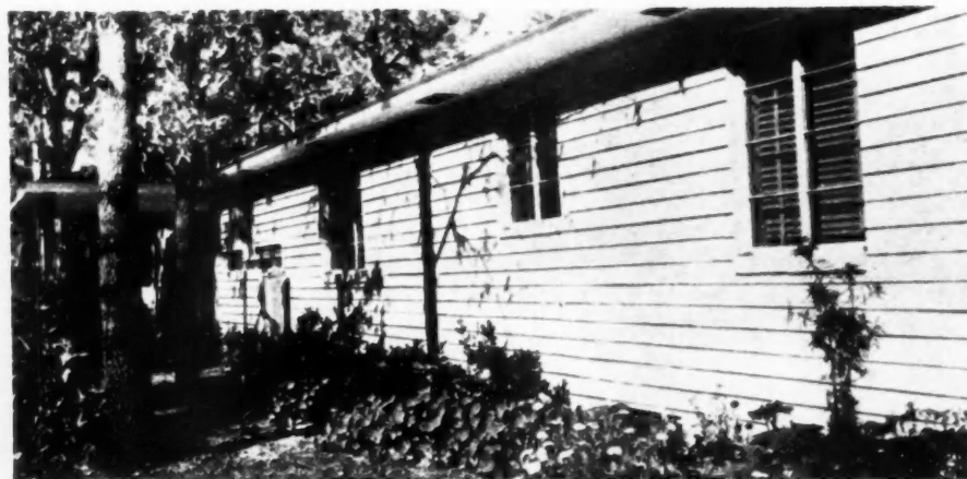
RAKING of horizontal joints and troweling others flush gave this special effect.
