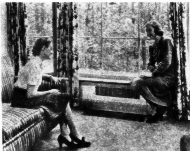
THERE is a trend toward the unit type of winter air conditioner. Air is drawn into the unit through the grille in the floor.
