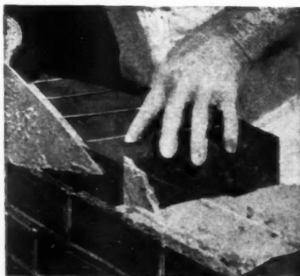
When a dab of mortar is spotted on one corner of the brick,
