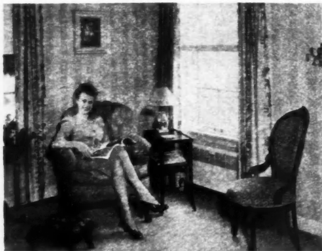
RECESSED convector radiation has been vastly improved in efficiency and appearance. The one shown is a typical installation.
