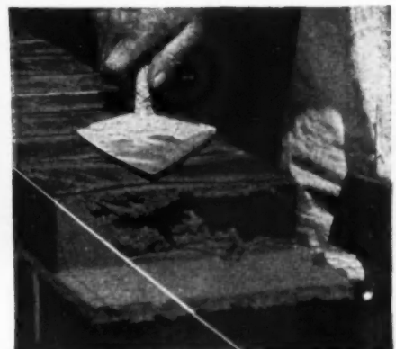
Slushing will not fill the voids.
