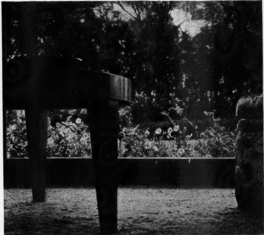
CONDITIONED AIR emerges from this grille below large living room windows to form a solid curtain between pane and room. Grilles under all other windows are at top of stool.
