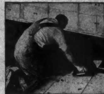
The panels provide an ideal surface for the application of whatever finished floor the owner chooses. Here the workman applies a mastic for linoleum or rubber tile. Likewise the floors provide an excellent base for hardwood or plywood and carpet.
