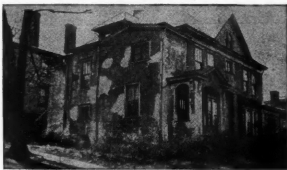
An example of disintegrated stucco surface on an otherwise well-built home and how the stucco was sealed, waterproofed and interior of home made dry with one heavy application of THOROSEAL.
