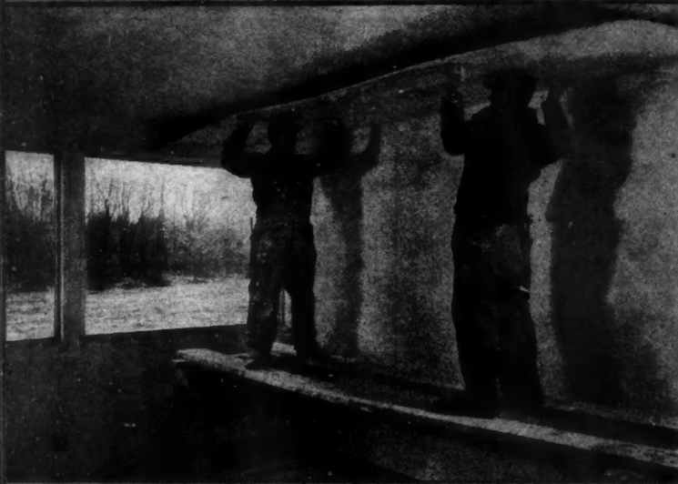
DRY WALL construction was used throughout the interior. Two thicknesses of \frac{1}{2} in. USG Sheetrock, the first course nailed vertically and the second glued horizontally, cover the walls over Fiberglas 3 in. blanket type insulation.
