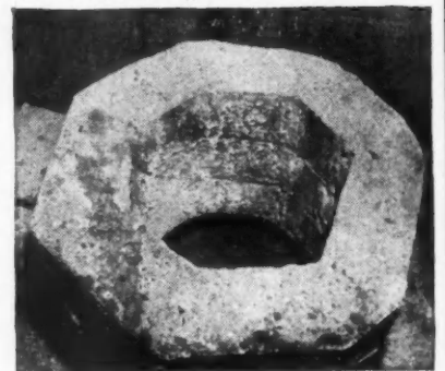
The sump pump well is no longer used. Pump was disconnected months ago. Water still rises to the floor level as can be seen in the above photograph — proving that the floor and walls of the pit are still surrounded by water held back by Aquella.
