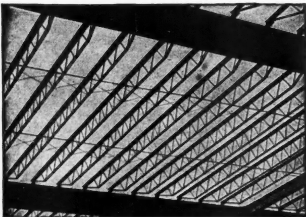
Simplicity of construction is made possible by Ceco steel joists. No skill is needed in placing them. They are easily moved into position and quickly spaced. After bridging, floor and ceiling are installed.
