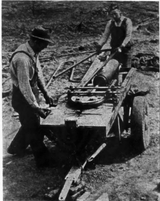
LOW-COST, cold bending of the wrought iron pipe that contributed to the over-all economy of the radiant heating system on this development, was accomplished by this home-made bending machine.
