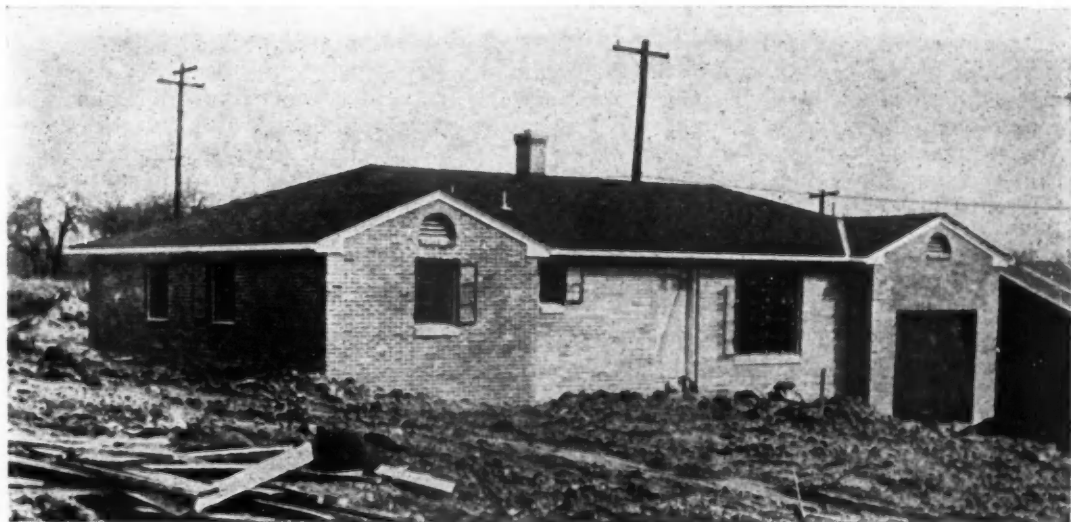
RIGHT: Partially finished exterior of one of the typical basementless, radiant heated houses in the first project of its kind in this country reveals a streamlined appearance. Cut stone is used on the front.
