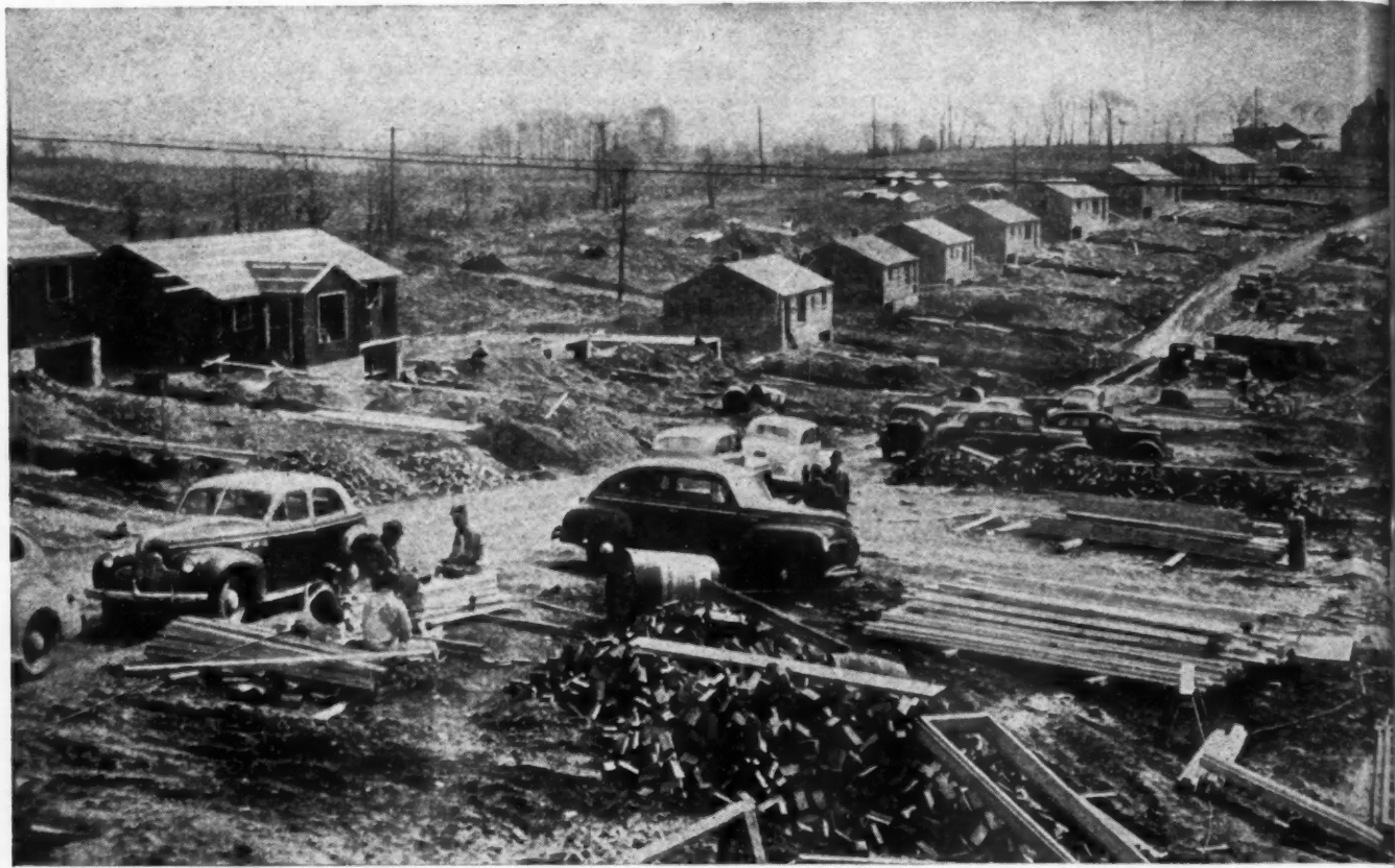
ABOVE: Shown under construction is a part of the Corace housing project which features radiant heating in each unit.
