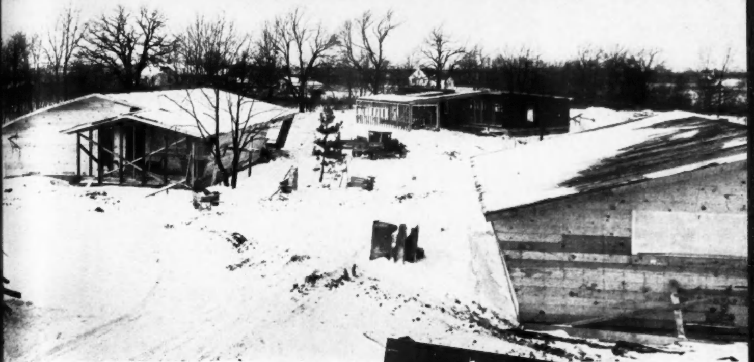
SHOWN under construction in the Ingersoll subdivision "proving ground" are two versions of house designed by Architect Alden B. Dow. House in right foreground is basic unit, one at left is expanded plan for wide lot.
