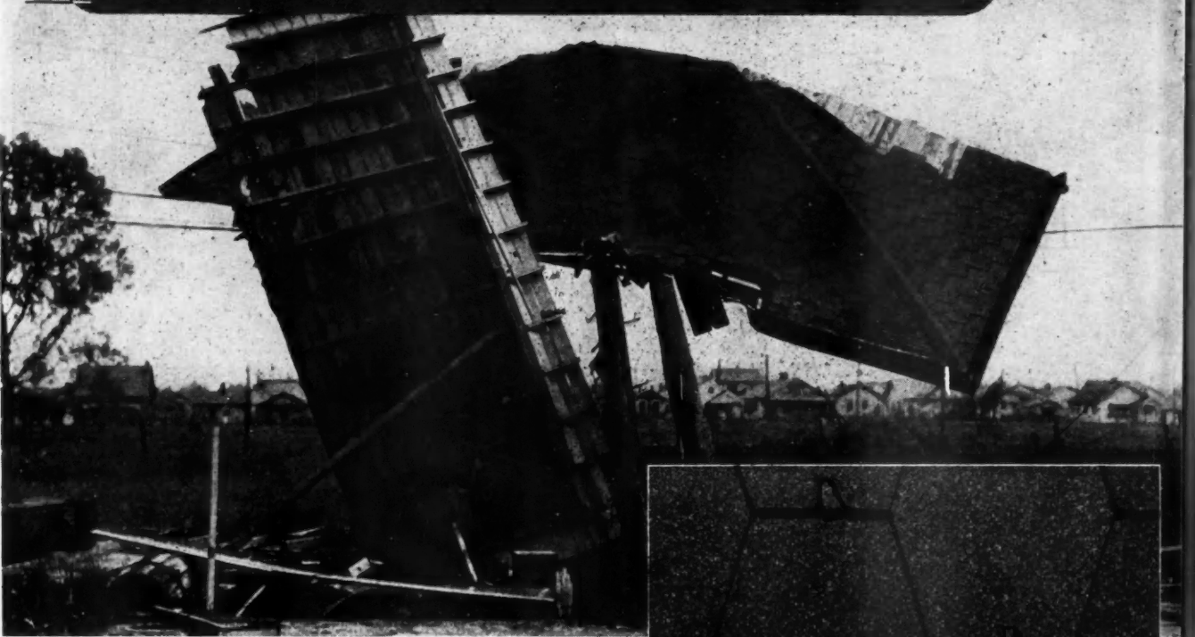
Photograph of roof deck blown completely off the house but with practically every Cyclone shingle intact.
