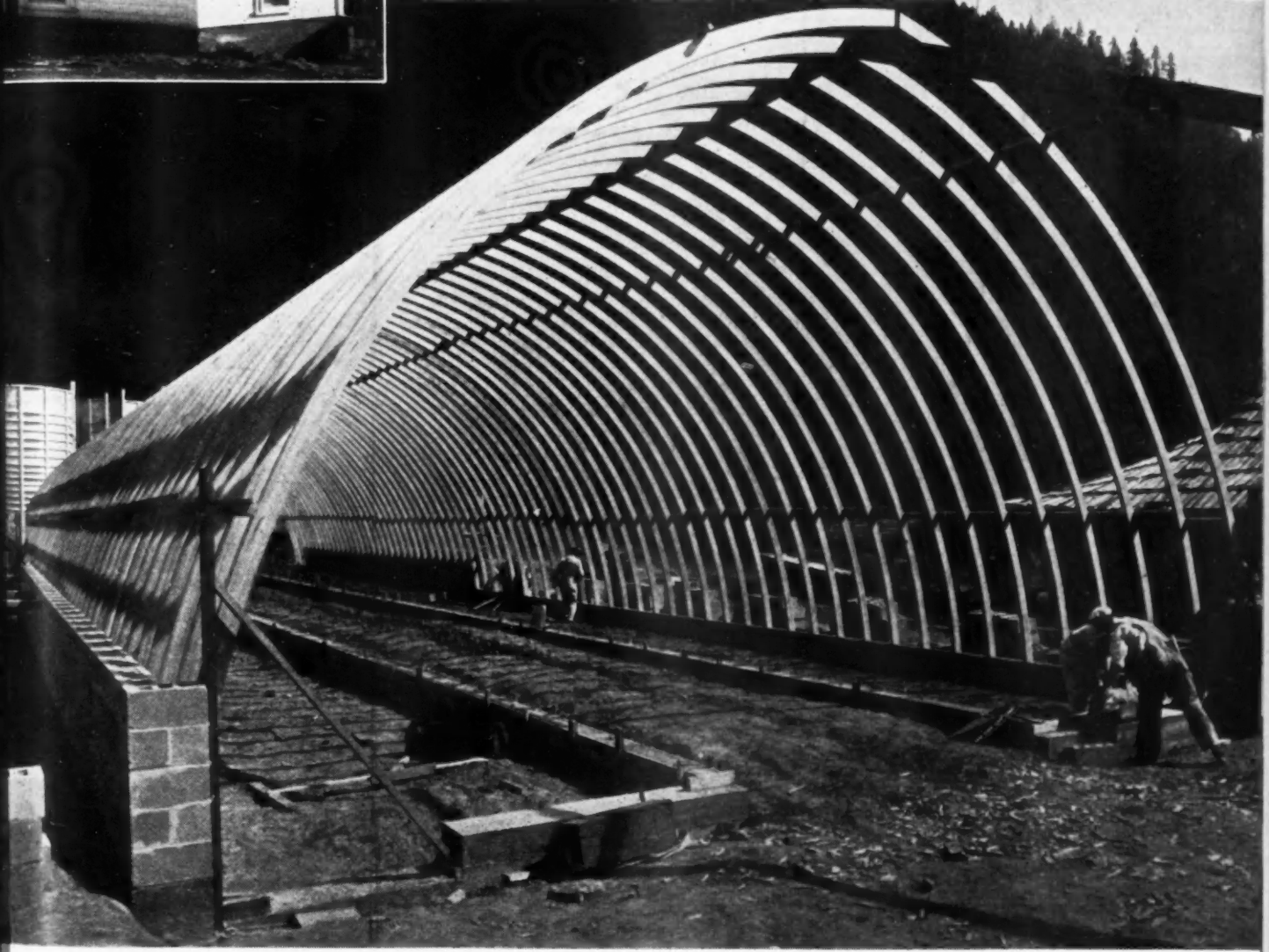
COW BARN under construction, showing curved laminated rafters on two foot centers.
