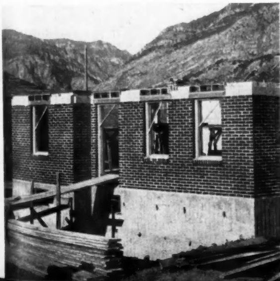
6 CLOSE-UP of job nearly ready for roof framing, pattern of vertical form boards shows.
