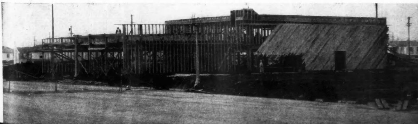
BELOW: Super-market under construction in shopping district which has stores, movie, bank, etc., grouped around central parking.
