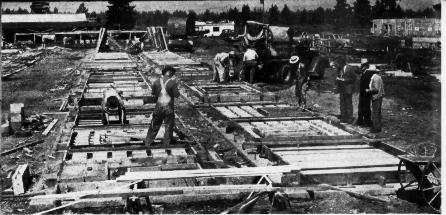
CARPENTERS setting up additional forms as the readymix truck fills others. Each panel is dimensioned and detailed accurately from blueprints to fit a definite place in a house. At upper left, formways recently cleared of panels and ready to start again.
