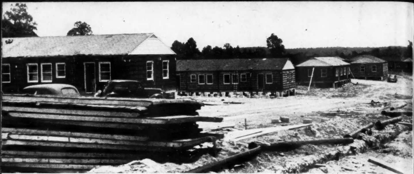
STREET VIEW of prefabricated housing units being erected on Alabama project after demounting and shipping from original site
