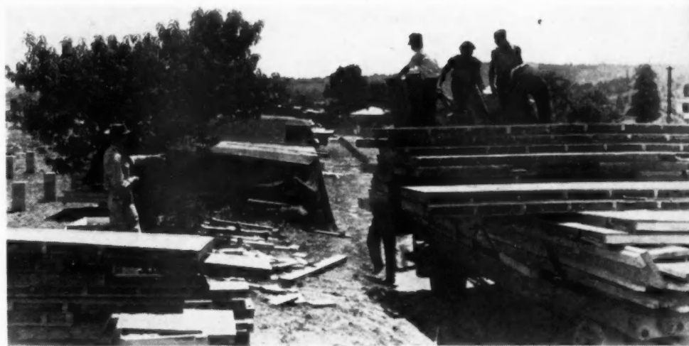
BELOW: Roof panels being re-erected; note two crews, one on ground, one on roof.
