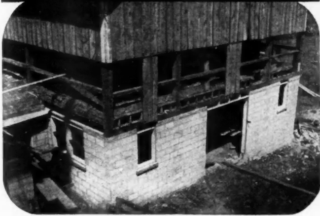
A sanitary concrete floor and new concrete masonry walls converted this old farm structure into a modern dairy barn. New concrete milk house (at left) was built at the same time.
