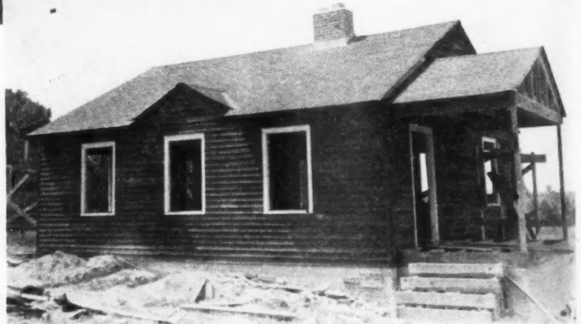
TYPICAL war housing by Sam F. Coleman, Anniston, Ala., on which siding was predipped in creosote using a trough and rack, as shown at the top of the page.
