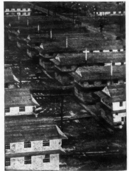
Construction of the 1,200 separate buildings at this cantonment, was speeded by the use of 600 barrels of Atlas High-Early cement daily. This shows a few of the buildings for which 30,000 cu. yds. of concrete for foundations was needed.
