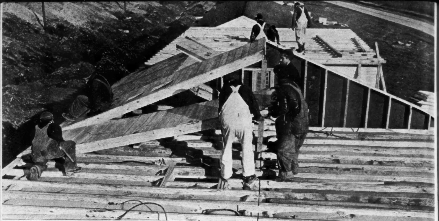
↑ ROOF SECTIONS built by Tonawanda, N. Y. lumber company are put in place by contractor Harry Stafford's crew at Dayton, O.
