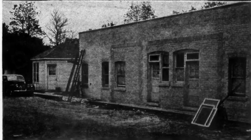
CONSTRUCTION VIEWS show sides where grease pit doors were replaced with bay windows for living rooms and entrances to the kitchens; when painted, old red brick trim was hardly noticeable. The V-pointed wings provide rear entrances to the kitchens of the two front units of this 4-apartment conversion project.
