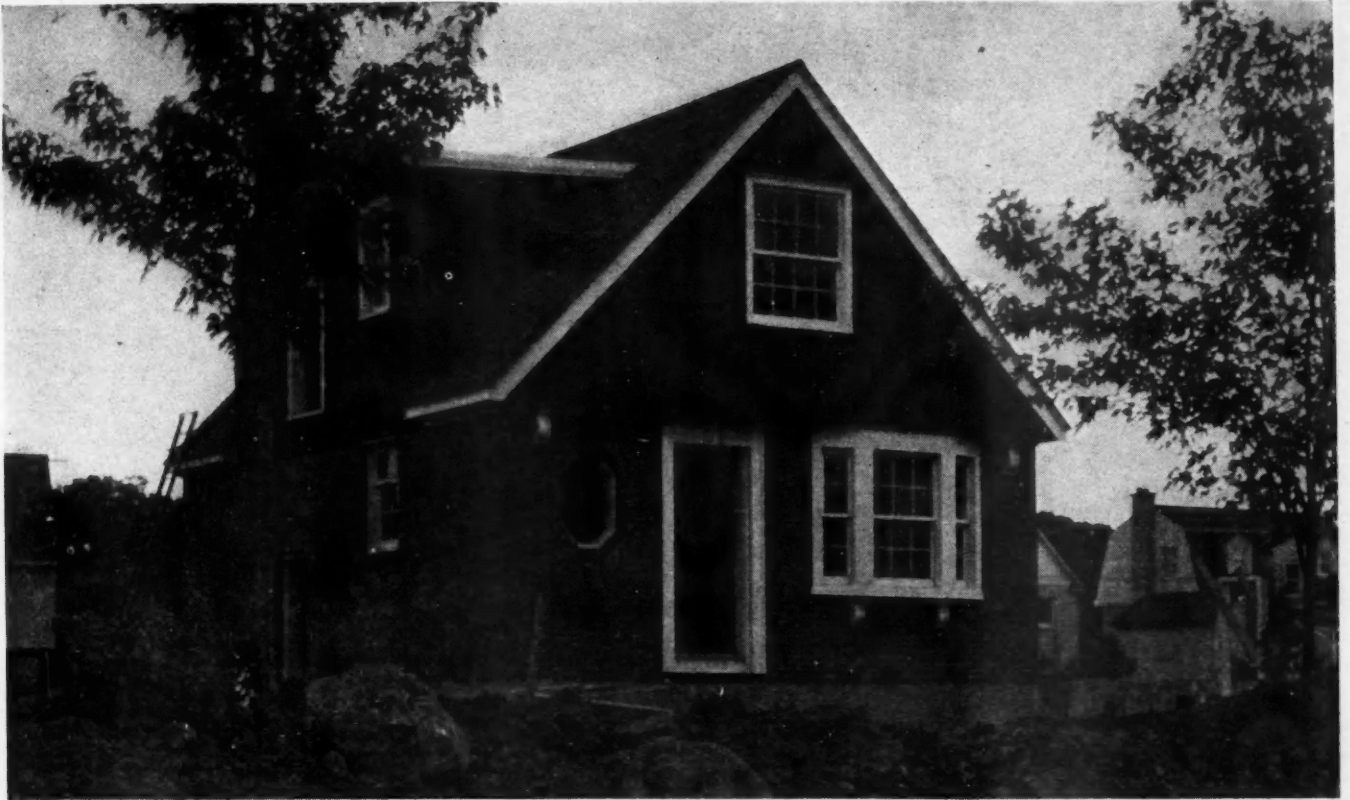
CONSTRUCTION VIEW showing a 1½-story war house of a street of similar units being built by Clairson Construction Co., in Ottawa.
