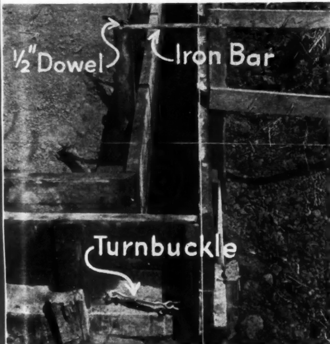
REMOVABLE FORM good for 100 foundations, built of 2 x 10's and 2 x 4's. Iron bars dropped across ½" dowels hold form rigidly in place. The form is quickly removed by kicking off the iron bars.
