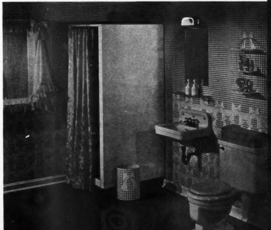
HERE is a typical bathroom planned for a war worker family in a converted building; non-critical materials are used in shower, lavatory and toilet.
