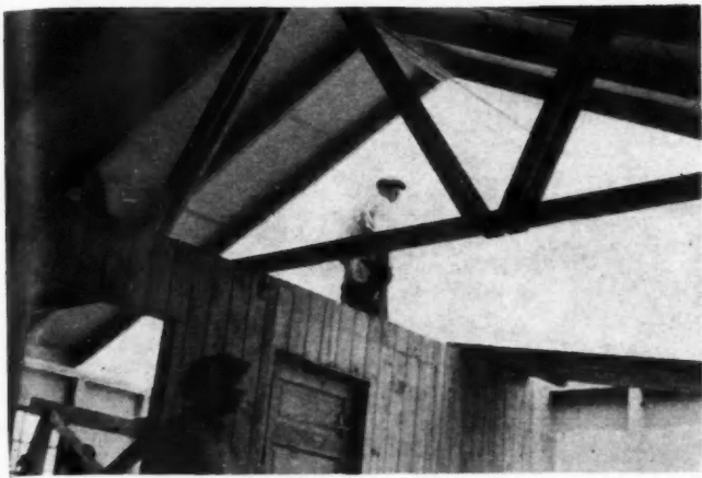
INTERIOR view showing trussed roof construction and inside partitions. Prefabricated truss members are assembled with bolts and split-ring timber connectors.
