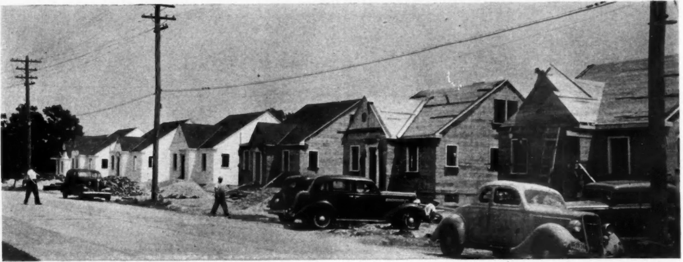
FAST WORK shown by private builders in erecting first group of FHA Title VI houses, at Bellmore, Long Island.
