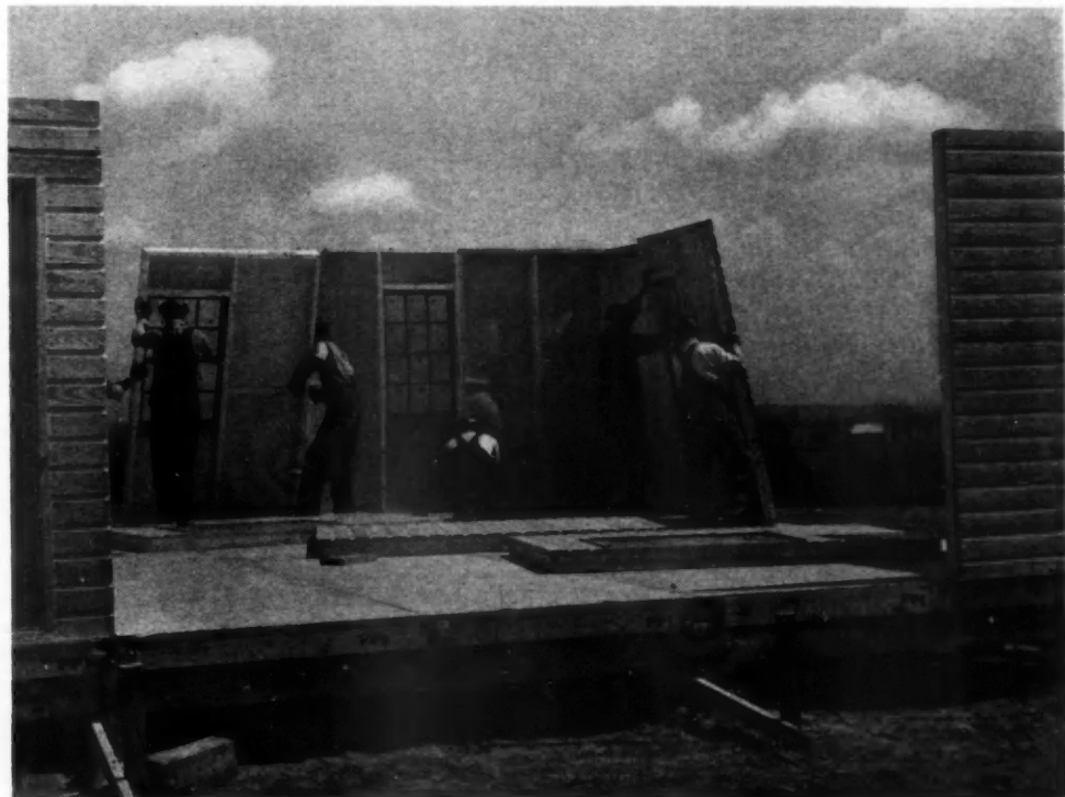
SETTING up the prefabricated wall panels after floor is in place. Panels are of southern pine drop-siding on 2 x 4's and are lined with insulation board. Panels are bolted together in assembly.
