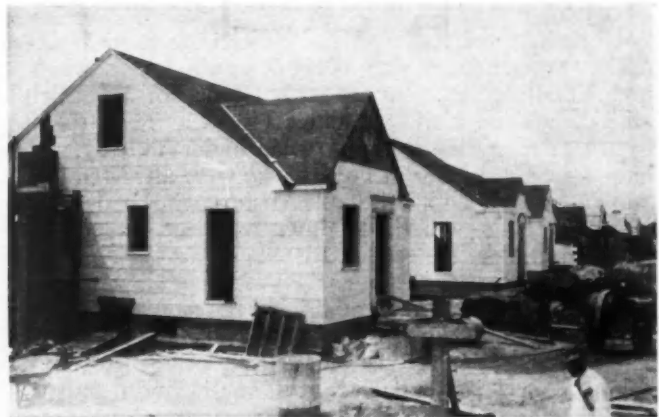
TITLE VI Bellmore houses under construction have 5-room 26' x 34' 6" plan as shown in drawing on the following page.
