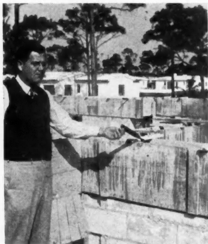
ON THE JOB, O'Dell points out metal rafter anchor to be imbedded in concrete beam.
