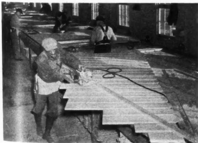
Electric handsaw trims off gable end assembly in National Homes shop; later to be set in place as one piece.
