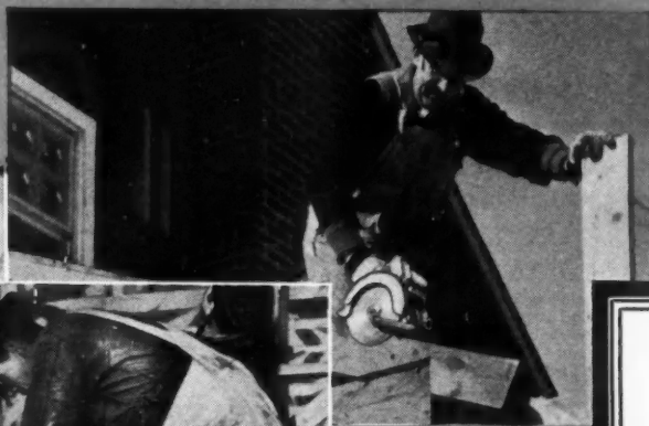
AT LEFT —Black & Decker No. 85 Electric QUICK SAW cutting off porch gable end. Note easy, one-hand operation of this popular model.
