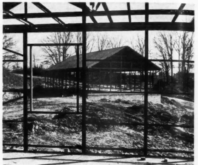
STEEL PANELS bolted together are used in two-family buildings for marines at Quantico, Va., seen under construction.
