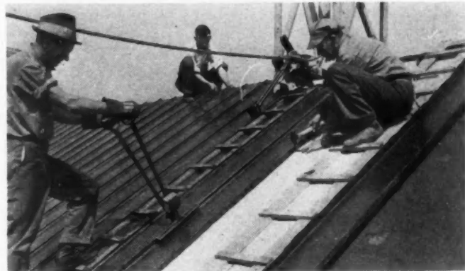
SOLDERING the cross seams on the old style terne roof was a considerable labor and maintenance expense, as indicated above. (Taylor Allderdice High School, Pittsburgh, Pa.) BELOW, a close-up of work on the Hooversen Heights school shows standing seam construction and illustrates the contrast between the former small sheets and the new long seamless strips.
