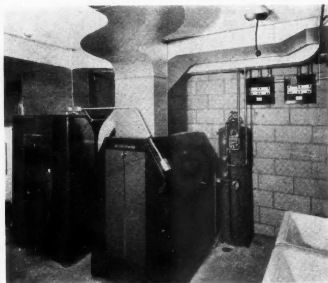
ANOTHER view of double heating system showing carefully planned and installed duct work.
