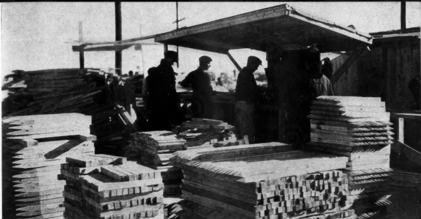
RADIAL SAW set up on job runs 24 hours a day to precut vast quantities of lumber used in building Camp Edwards barracks.
