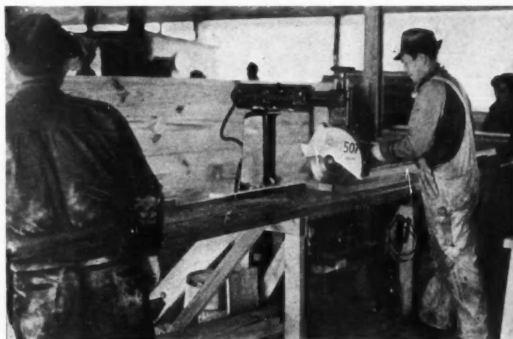
ONE OF A BATTERY of radial saws in central cutting station where stairs, steps, brackets and trim are turned out very rapidly.
