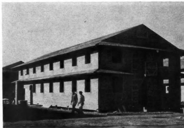
TYPICAL BARRACK is two stories high, has winter air conditioning plant, and houses 63 men. Interiors are lined with gypsum board.
