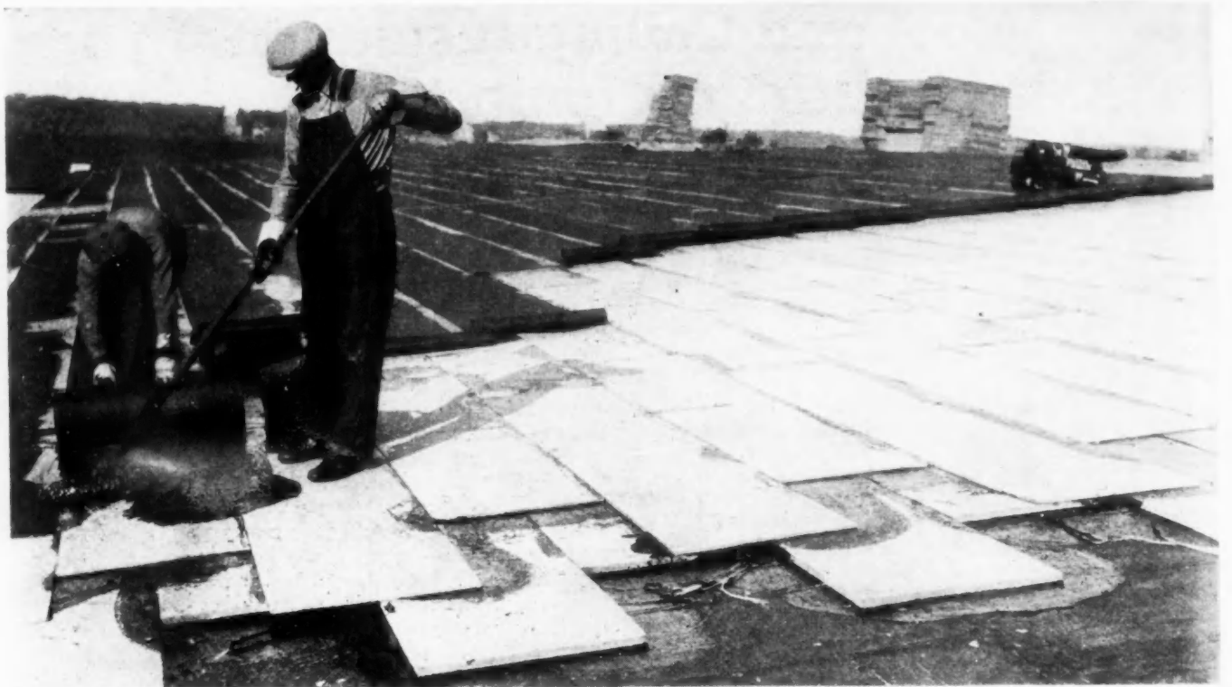
ROOF INSULATION Board being applied in two layers in hot asphalt on large industrial plant at Ottawa, Ill.; C. R. Dick, Architect.
