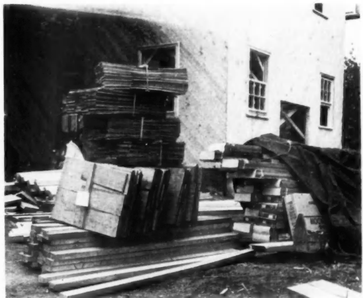
KILN-DRIED PACKAGED LUMBER and endless sheathing are used. Note care with which packaged lumber and frames were covered with tarpaulin. (Tarpaulin was in this case temporarily turned back for photographing.)
