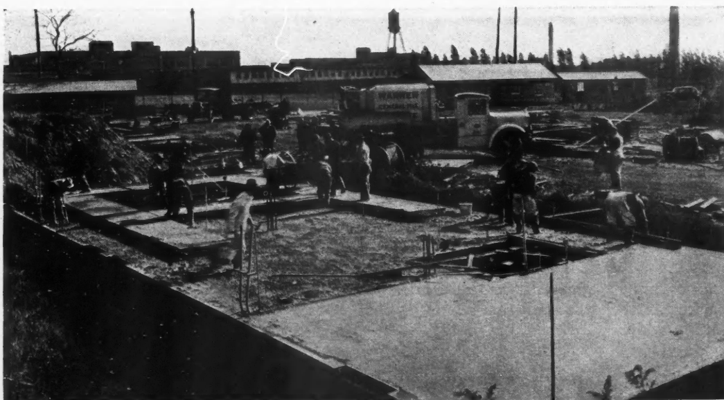
POURING and screeding concrete for the first floor of a structure in the Philadelphia Hill Creek Housing Project. Calcium chloride was used to speed up the setting as an added cold weather precaution.
