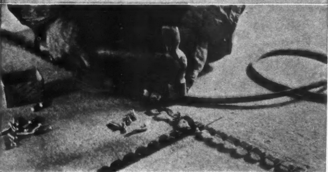
SETTING the runner strips for steel partition studs in the Ten Eyck Homes. Holes were electrically bored in the concrete and the strip anchored with "Rawl-Drives."
