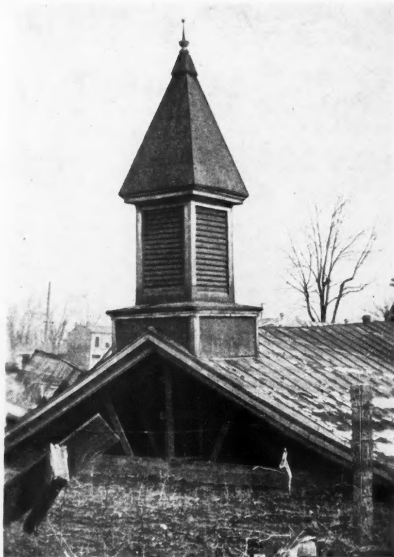
THIS church roof of timber construction still structurally intact, had floated off the brick walls for lack of sufficient anchorage.
