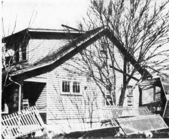
ORDINARY good construction of toenailing studs to sills, and bolting sills to foundation, prevented dislodgment of this bungalow, although it has been exposed to a swift current and submersion.
