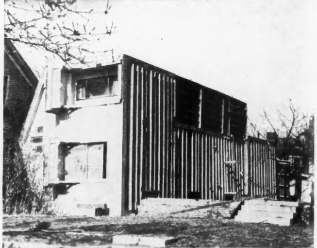
THE OVERTURNING of this house was caused by high flood waters, swift current, and lack of anchorage to the brick foundation.
