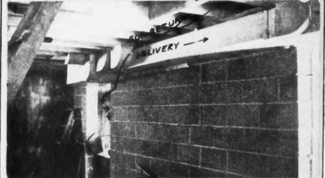
FIG. 4 SAME BASEMENT BUT TO THE LEFT OF DIVIDING WALL. NOTE COMPACT WARM-TRUNK. RETURN-AIR DUCT WILL LIE PARALLEL.
