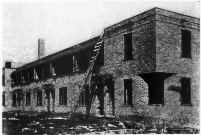
CONSTRUCTION view of court units in Beverly Hills project. Note separate entrance and covered sun porch for each apartment.
