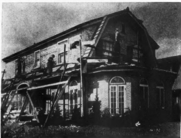
OVERCOATING —view showing modernizing of an old house with sheet material that looks like brick. A number of low cost overcoatings of this type are available.
