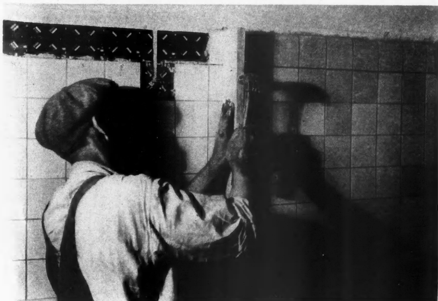
Ceramic Tile Clipped to Metal Lath Is Inexpensive to Install, and Does Not Crack.
