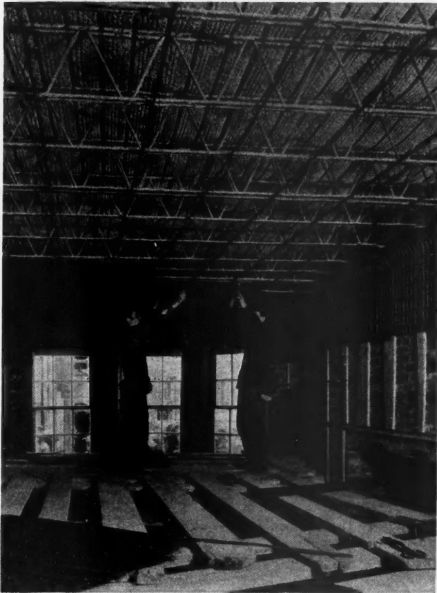
All Floors Are of Concrete and Metal Lath Construction Supported by Bar Joists.
