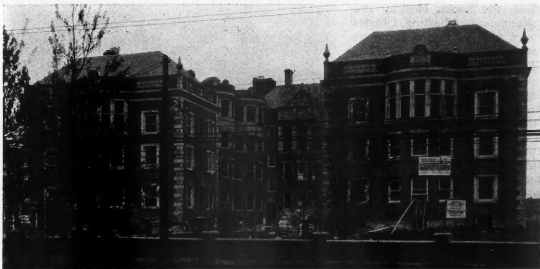
The Leeb-Tyroler Apartments, 16000 South Morland Blvd., Shaker Heights, Ohio, Showing Progress of Construction on May 12, 1931.
