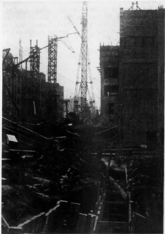
For some units a pile foundation was used with a reinforced concrete footing placed on top.
