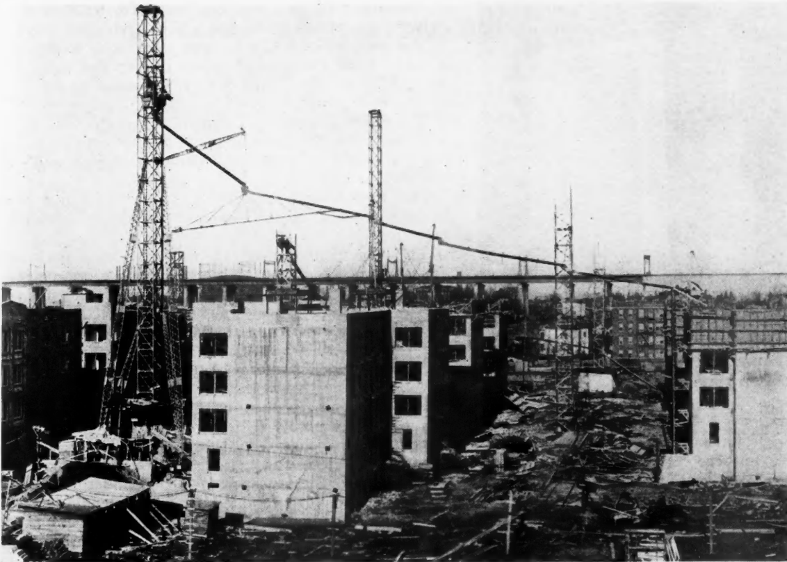
The unit in the foreground to left is the building that started to tip over.
