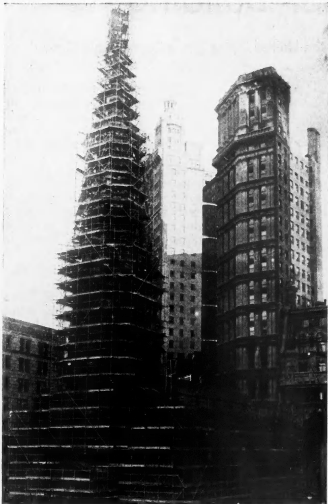
In Restoring Historic St. Paul's Chapel, New York, Steel Scaffolding and Flameproof Wood Platforms Were Used.
