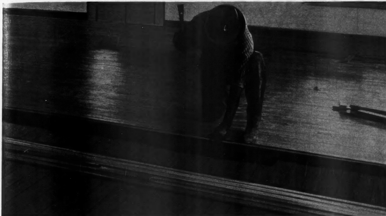
Oak Flooring of Various Sizes and Grades Can Be Laid Over Worn and Obsolete Floors with Results Equal to Oak Floors Laid in New Construction and Such Work Offers the Contractor an Important Field of Work, Especially in Winter When Work Is Needed to Hold the Organization Together.
