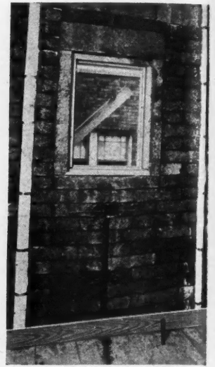
Space for Large Pipes Is Provided During Construction While Small Pipes Are Set by Raking Out a Depression.
