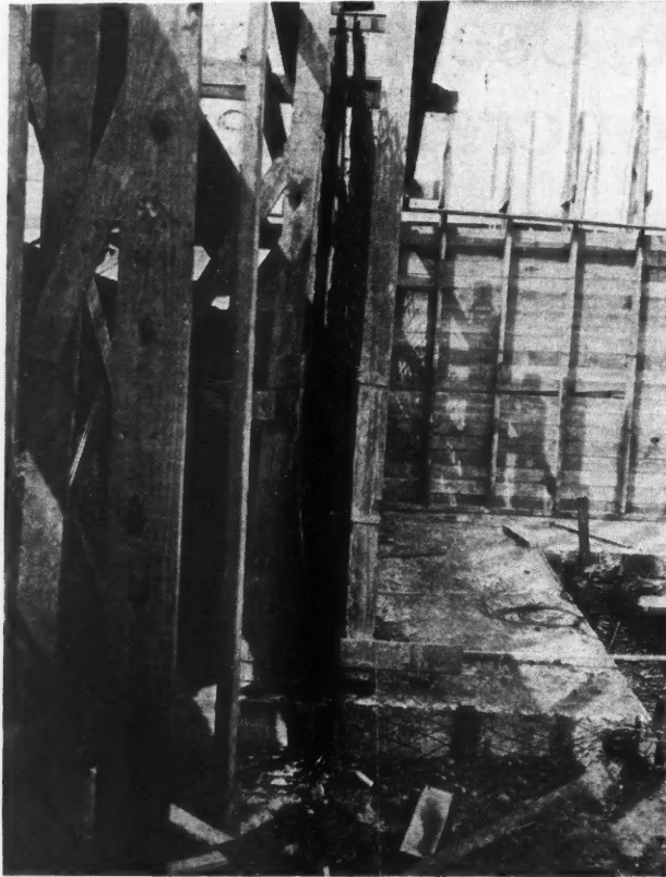
Fig. 3. Expanded Metal Has Proved Adaptable to the Reinforcing of Concrete Walls of Swimming Pools and Reservoirs.
