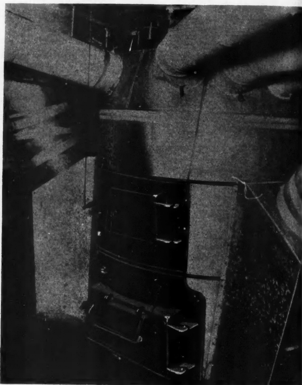
Warm Air, Central Heating Plant with Over-head Type Motor-fan Unit, Motor Suspended on an Arm Extending from an Iron Standard on the Left Side. On either side of the front are cold air intakes of a type becoming standard except where there is a rear fan.
